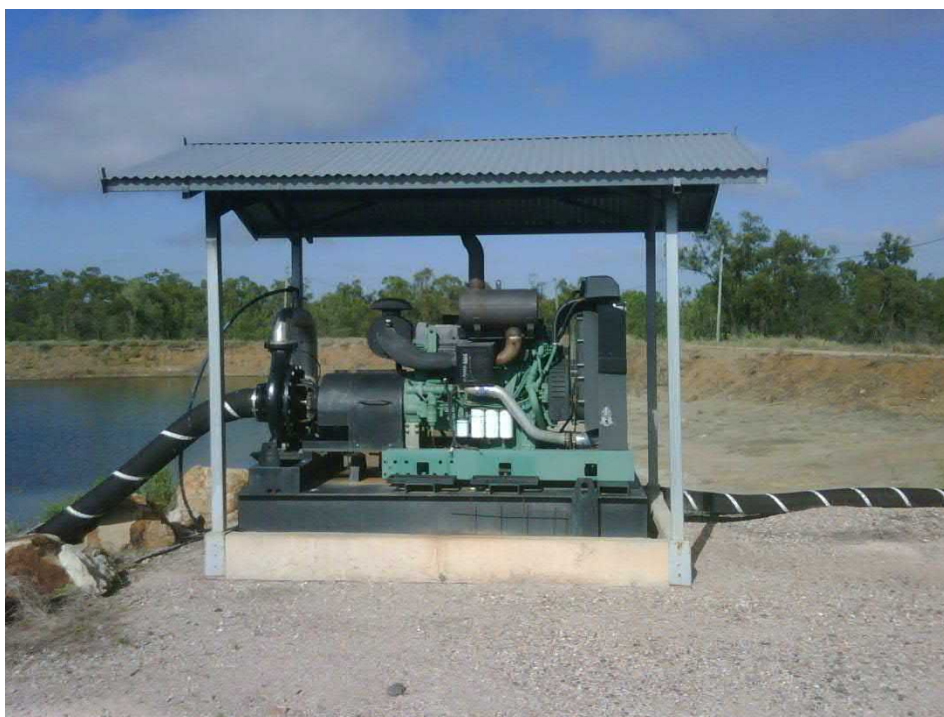
Settlement Dam diesel pump
