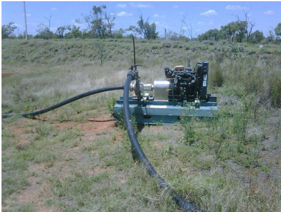
Mt Hope Extension Dam diesel pump
