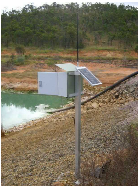
Typical dam automatic monitoring station
