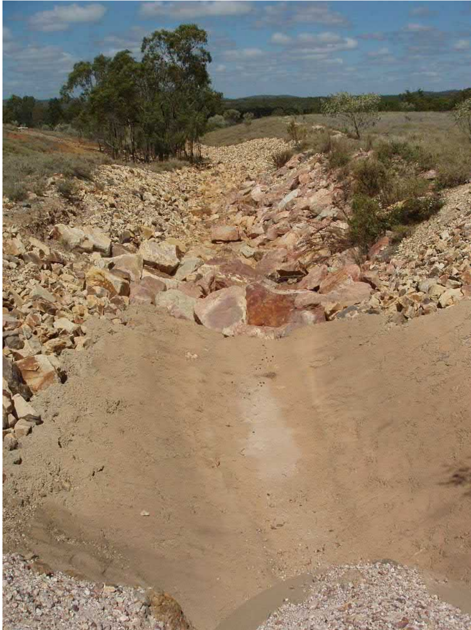
Inflow drain to Settlement Drain
