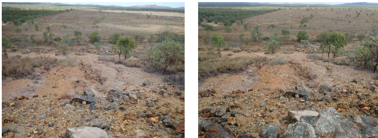
Figure 3-25: An erosion gully on the Southern WRL Batters in 2019 (left) and 2020 (right)
