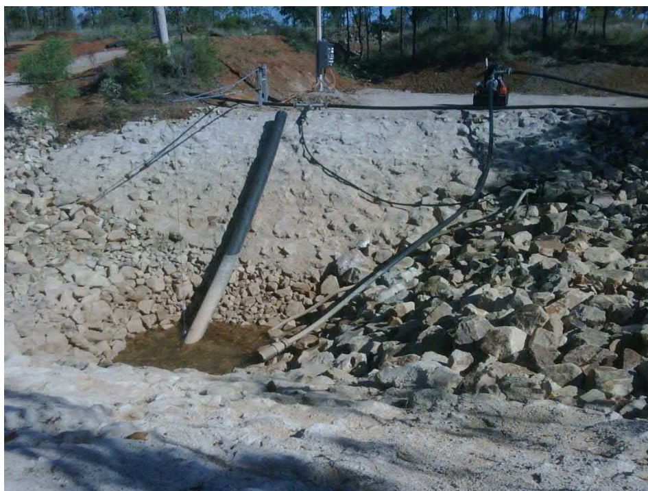
Mt Mawe Dam Sump diesel pump
