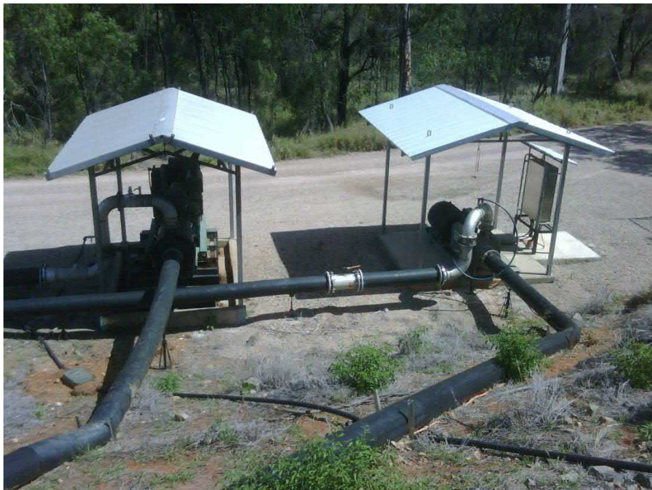
Mt Hope Dam electric and diesel pumps
