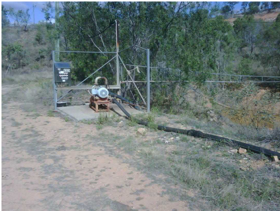
ONTD N Sump electric pump
