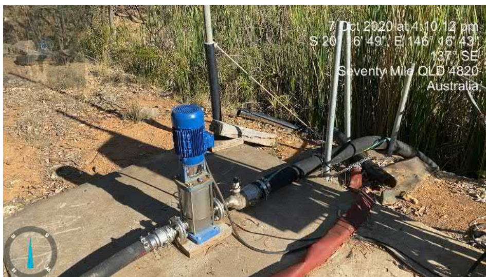
Raw Water Dam Solar Pump
