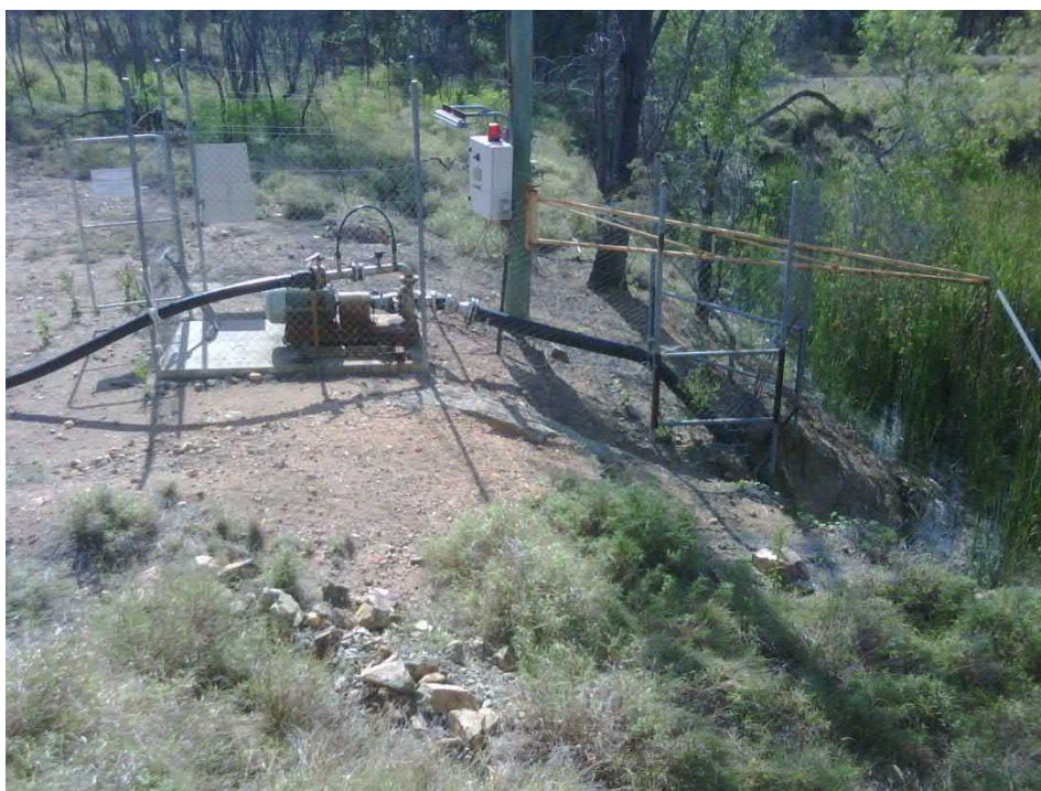
NNTD W Sump electric pump
