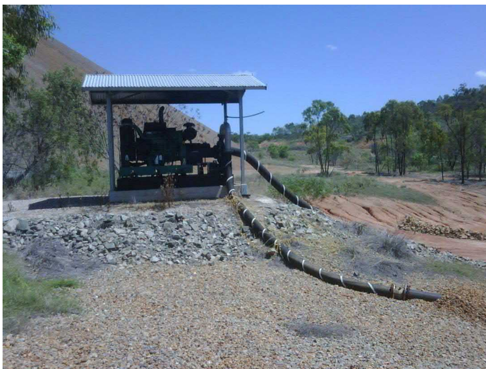
Plum Tree Creek Dam diesel pump
