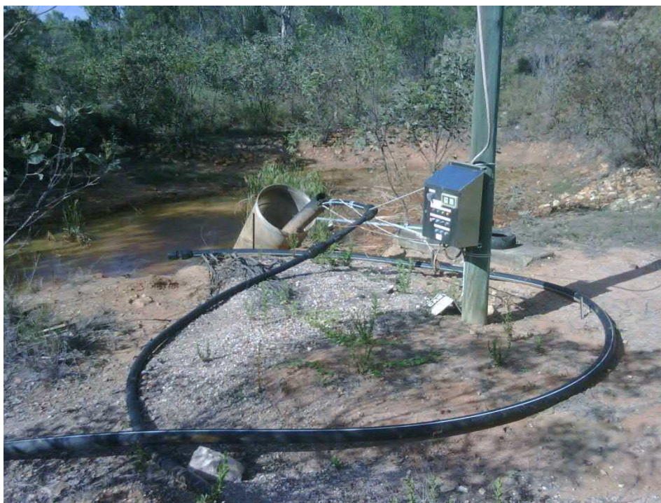
ONTD E Sump electric pump (submersible pump)
