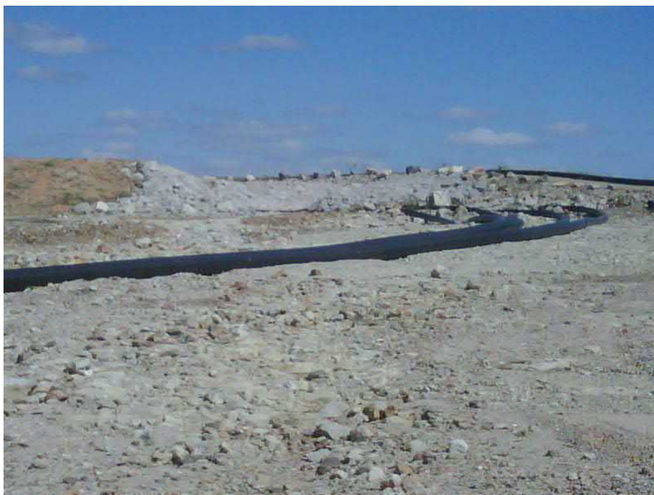
Eastern Waste Rock Dump low flow bypass facility
