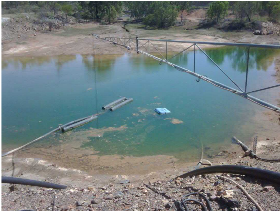
Supergene Dam electric pump (submersible pump)
