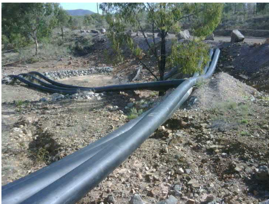
Supergene Stormwater Dam low flow bypass facility
