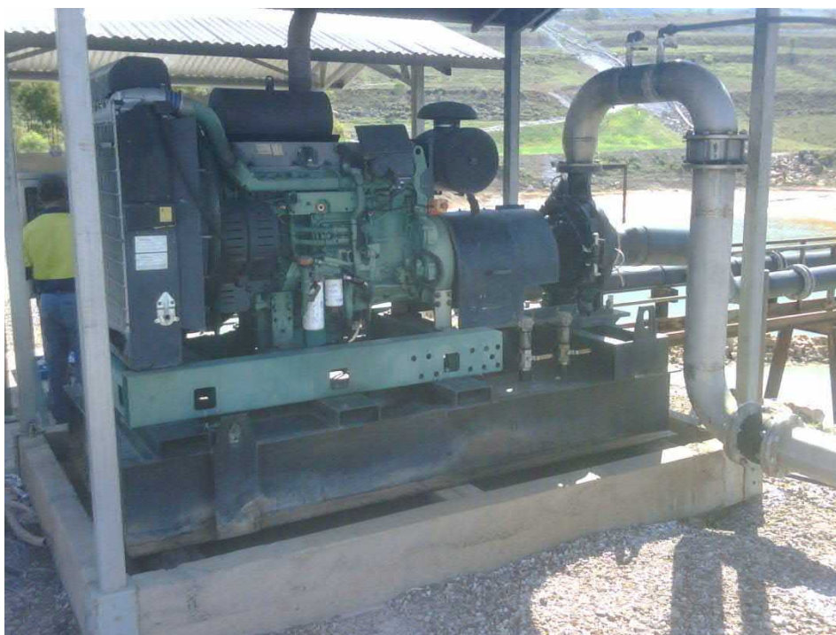
Mt Mawe Dam diesel pump
