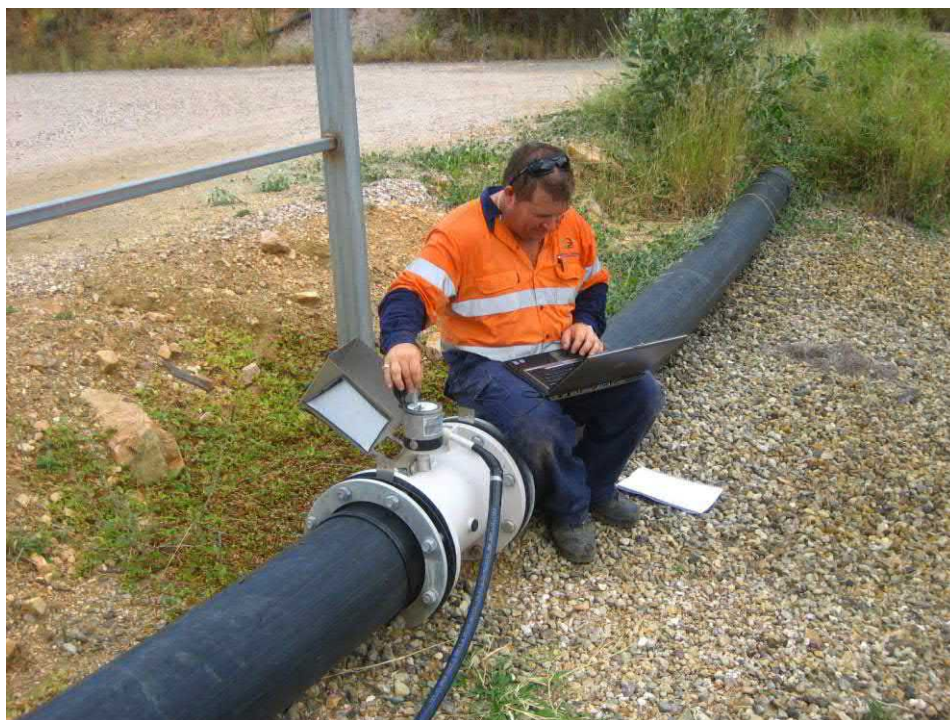
Typical dam automatic monitoring station – flow meter on pump discharge pipeline
