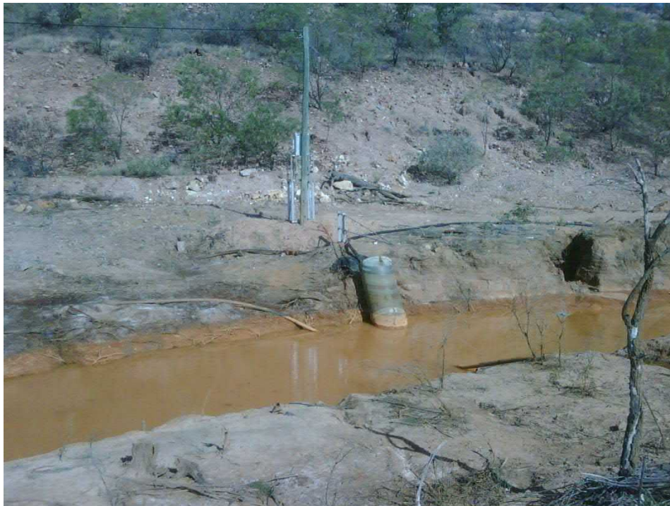
ONTD W Sump electric pump (submersible pump)
