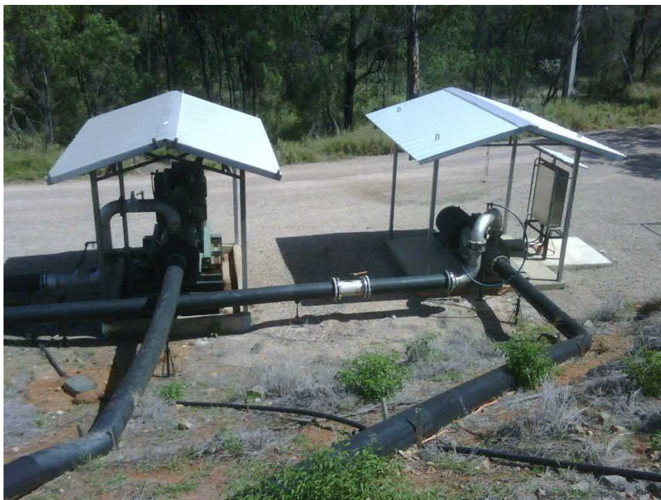
Mt Hope Dam electric and diesel pumps
