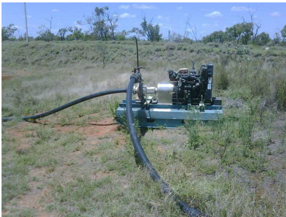
Mt Hope Extension Dam diesel pump
