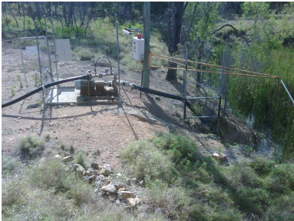
NNTD W Sump electric pump
