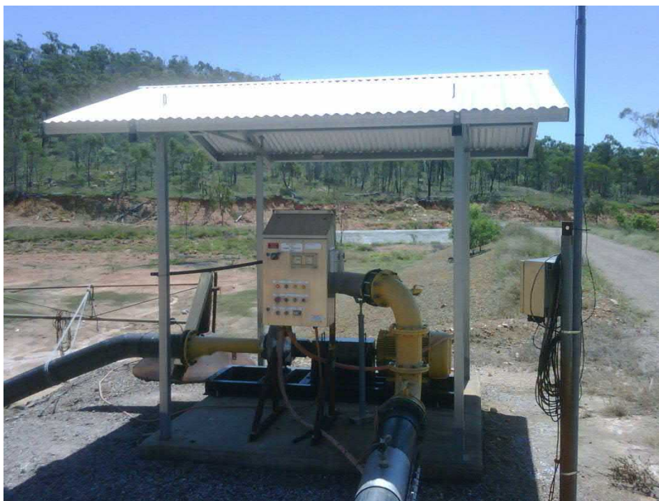
Plum Tree Creek Dam electric pump
