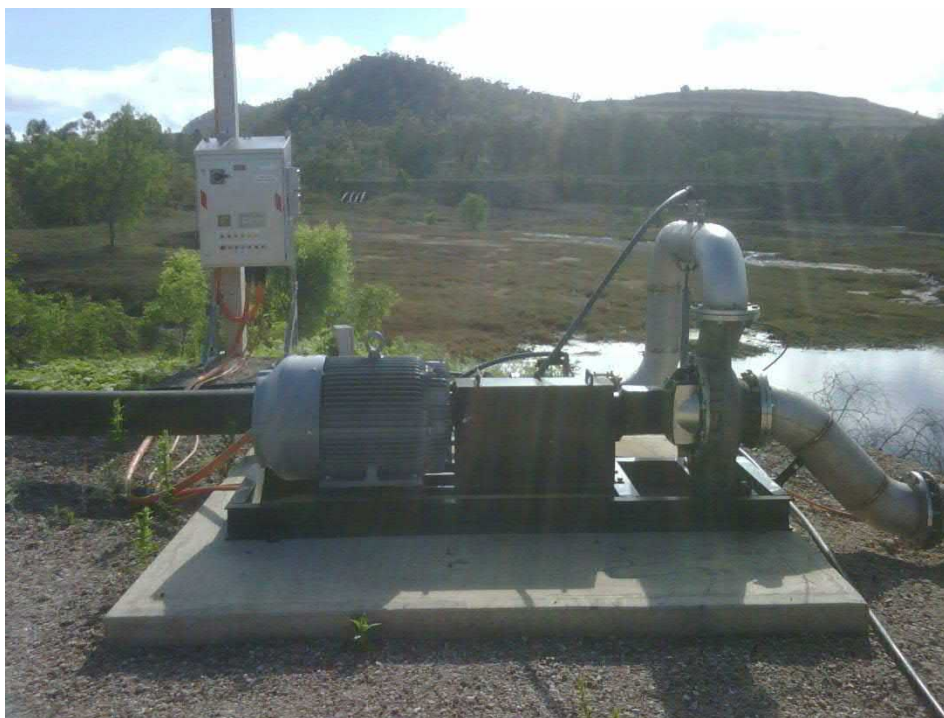
Settlement Dam electric pump
