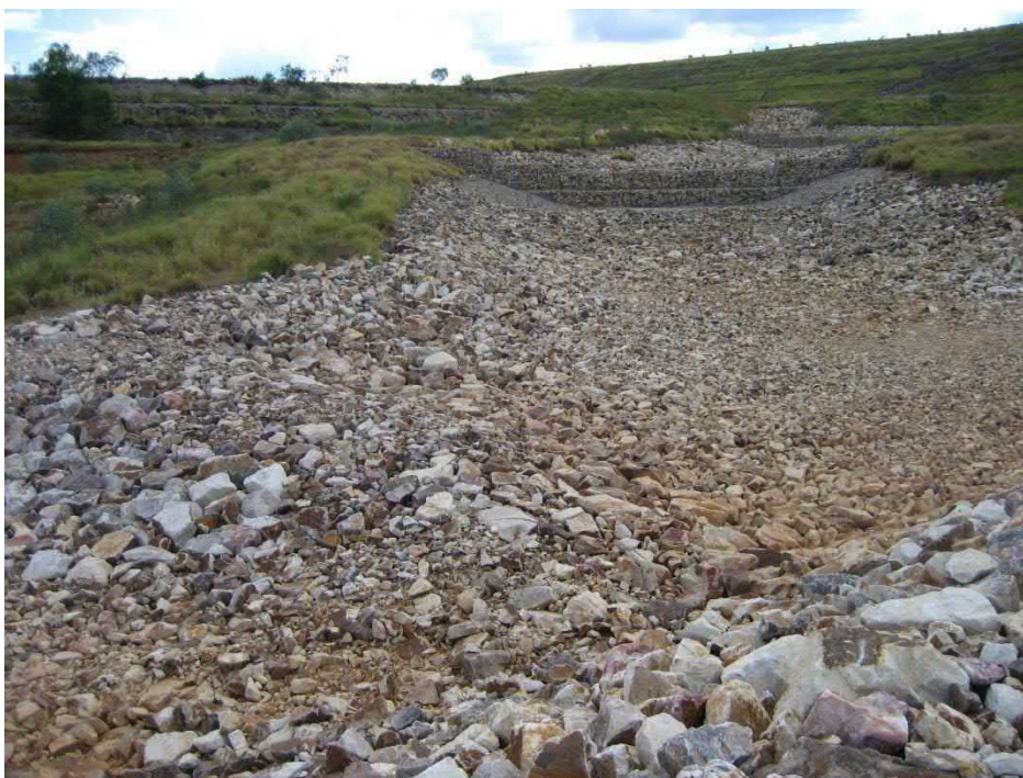
Mt Hope Dam high flow bypass facility
