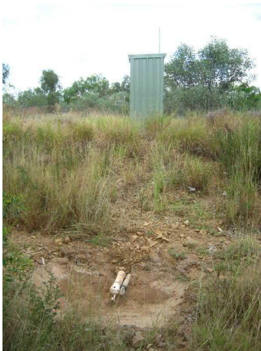
Mt Hope Dam high flow bypass automatic monitoring station
