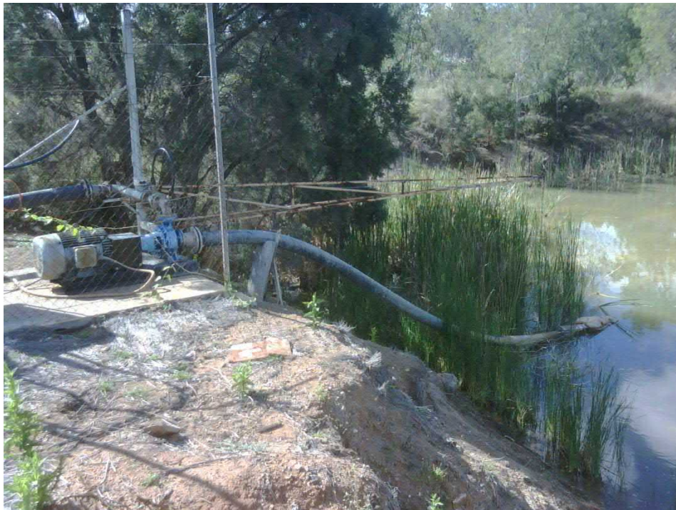
NNTD N Sump electric pump
