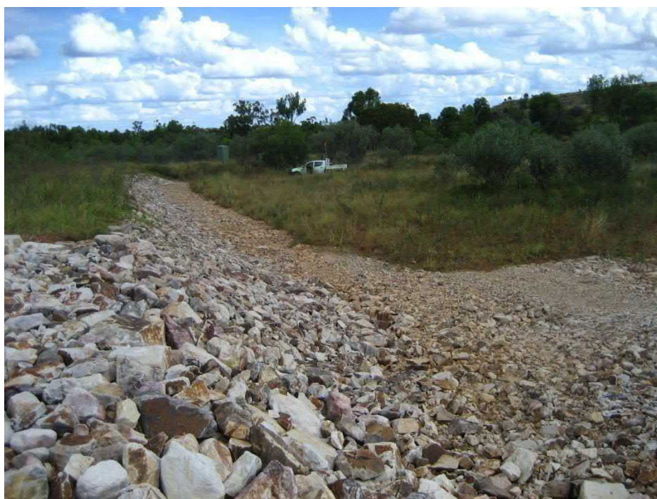
Mt Hope Dam high flow bypass facility
