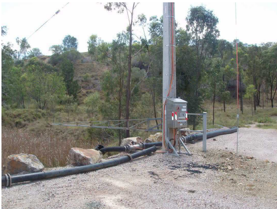
STD SW Sump electric pump (submersible pump)
