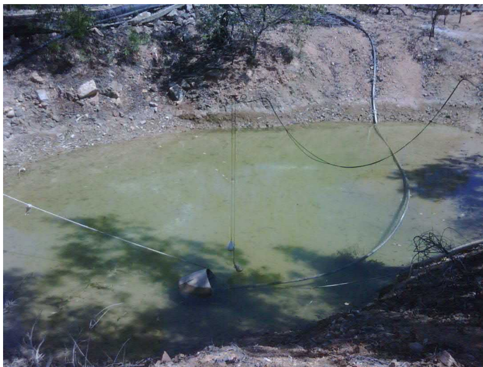
Supergene Stormwater Dam Sump electric pump (submersible pump)
