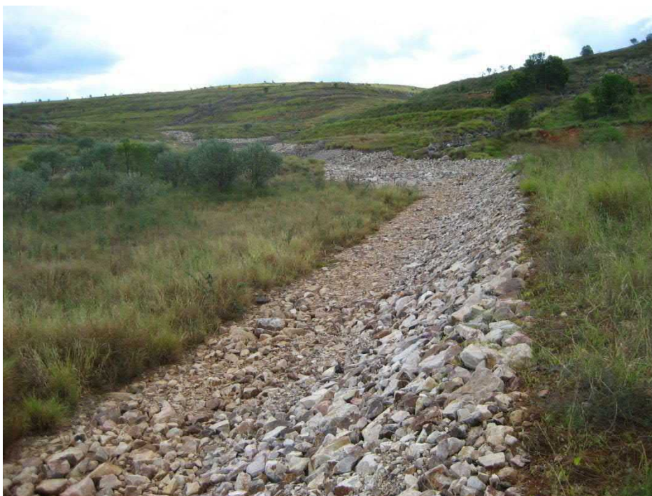
Mt Hope Dam high flow bypass facility
