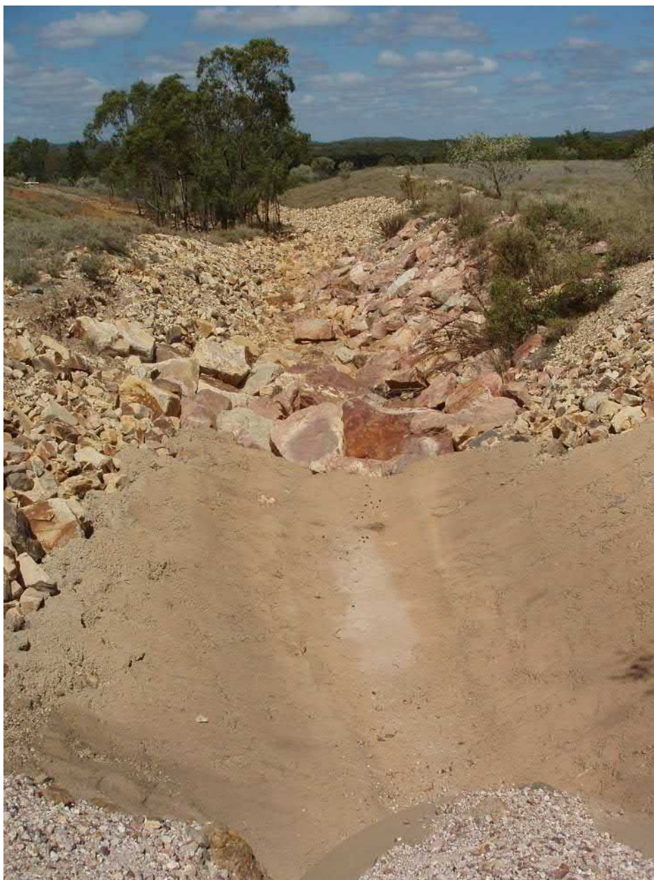
Inflow drain to Settlement Drain
