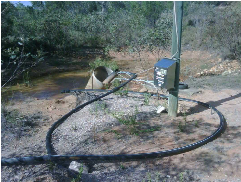
ONTD E Sump electric pump (submersible pump)
