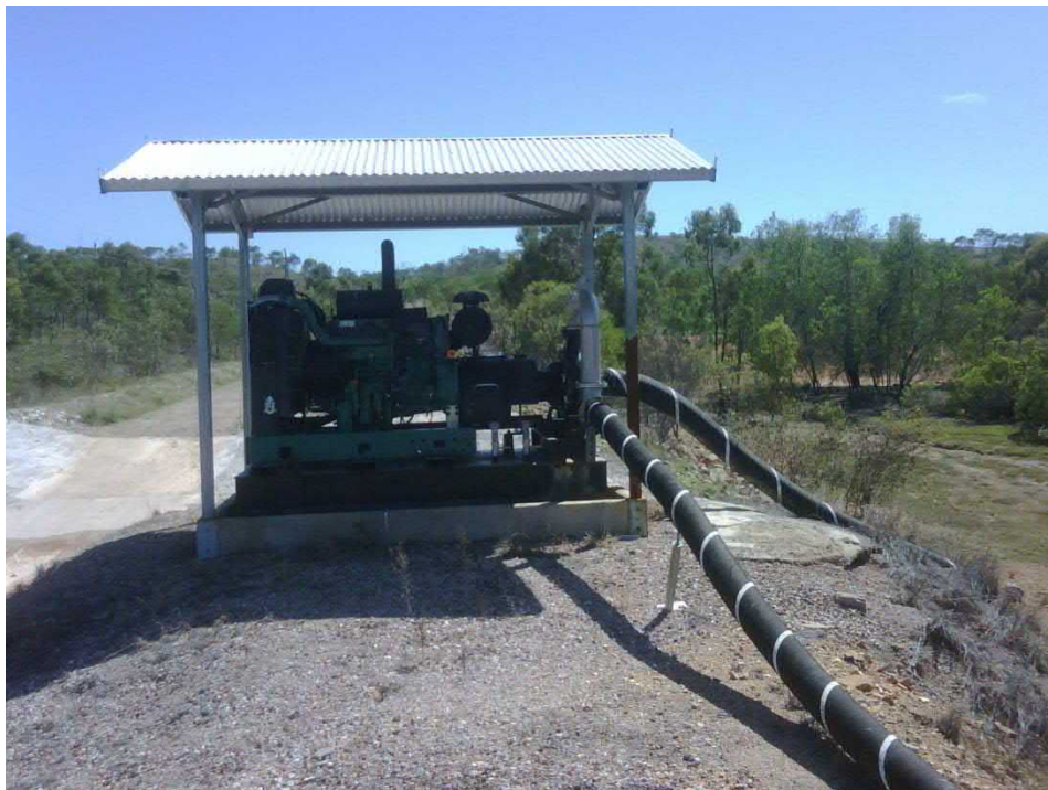
Supergene Dam diesel pump
