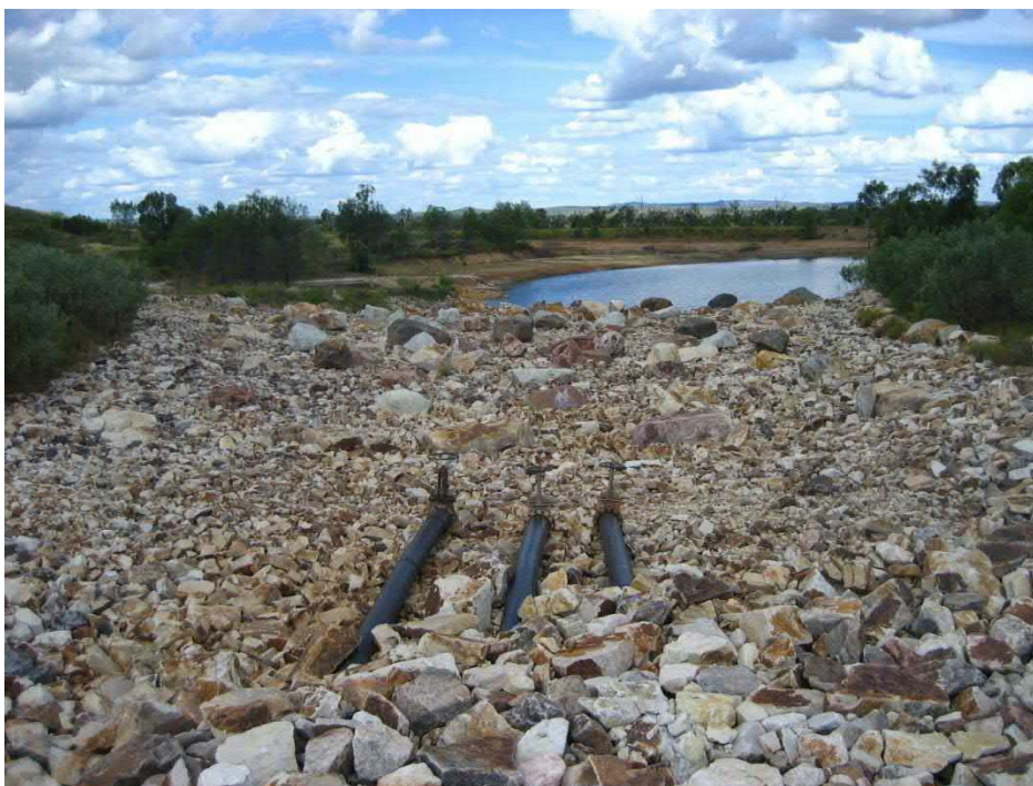
Mt Hope Dam high flow bypass facility
