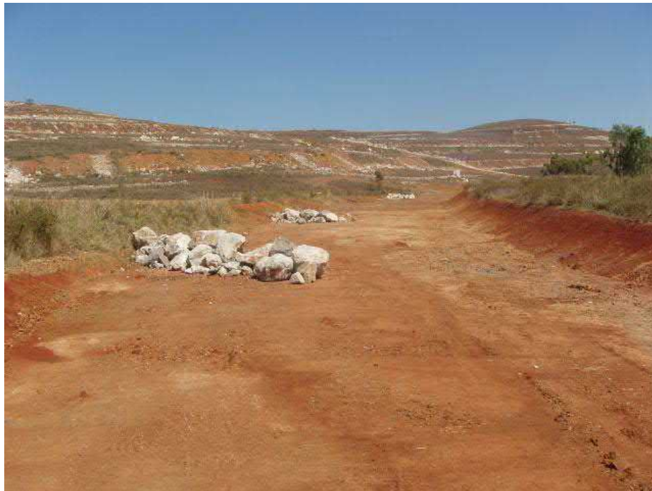
Golden Star Pit diversion channel around Mt Mawe Dam
