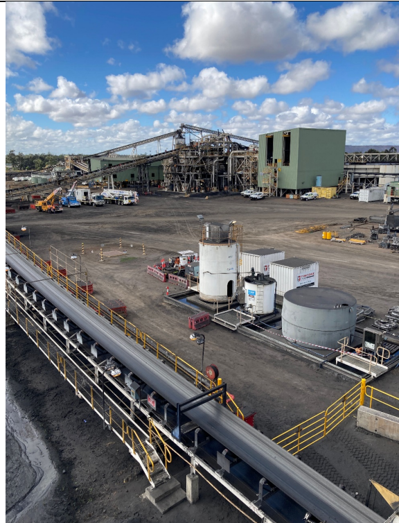
6. CHPP Infrastructure and bulk flocculant storage tank in foreground
