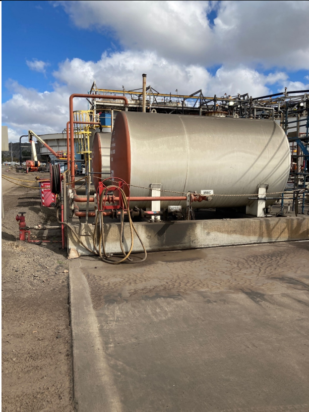
9. Bunded delivery pad – subsidence noted in the center of the photo
