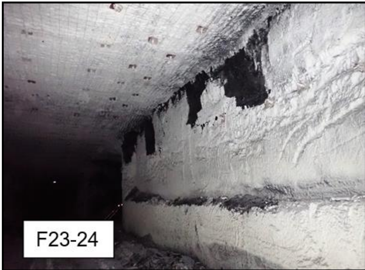
Figure 31. Typical Thin Rib Spall at Ensham after Secondary Coal Recovery – F23-24, 109A Panel
