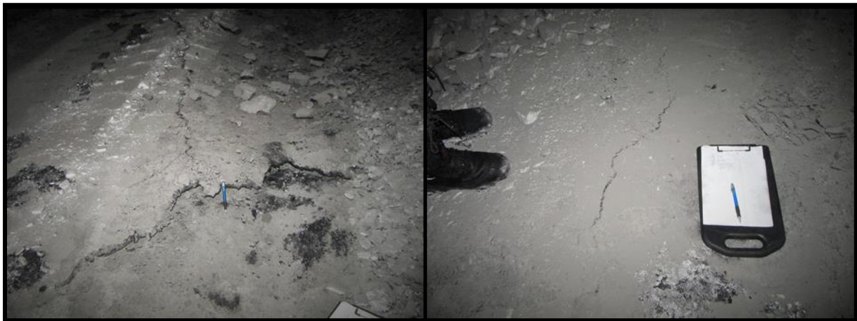
Figure 33. Minor Cracking of the Coal Floor, 101 Panel
