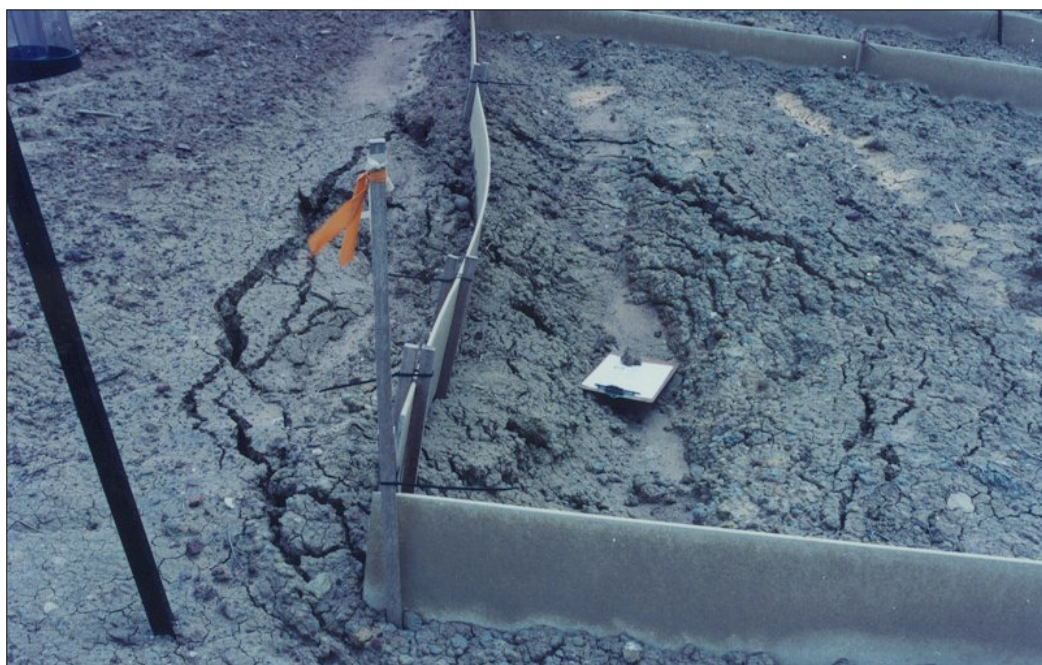
Photo 12: Slumping on the 30% spoil plot, 1994.
