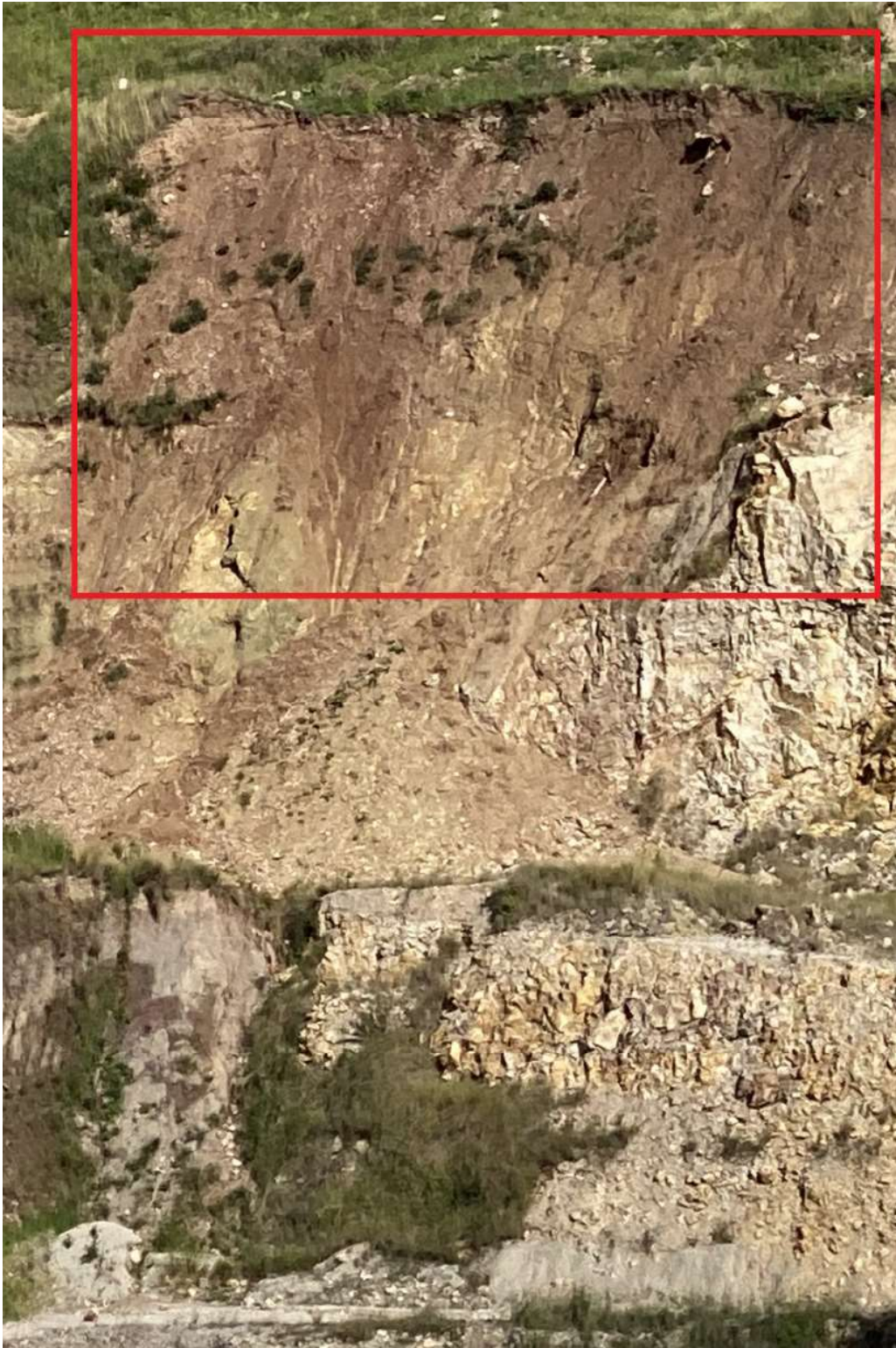
Figure 9. Typical bench scale rotational sliding failure through weathered andesite on the north wall.
