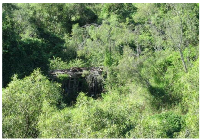
Figure 2.12 Deteriorated abandoned rail carriage
