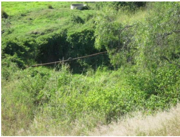
Figure 2.11 Washed out rail bridge
