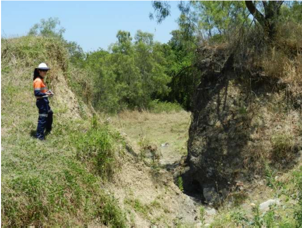
Figure 2.2 Failed detention dam discharging offsite
