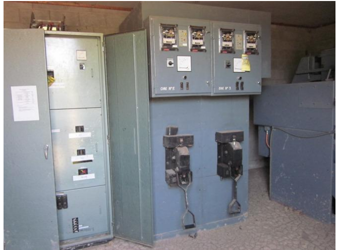
Photograph 48 – Old electrical equipment now decommissioned (15/11/11).
