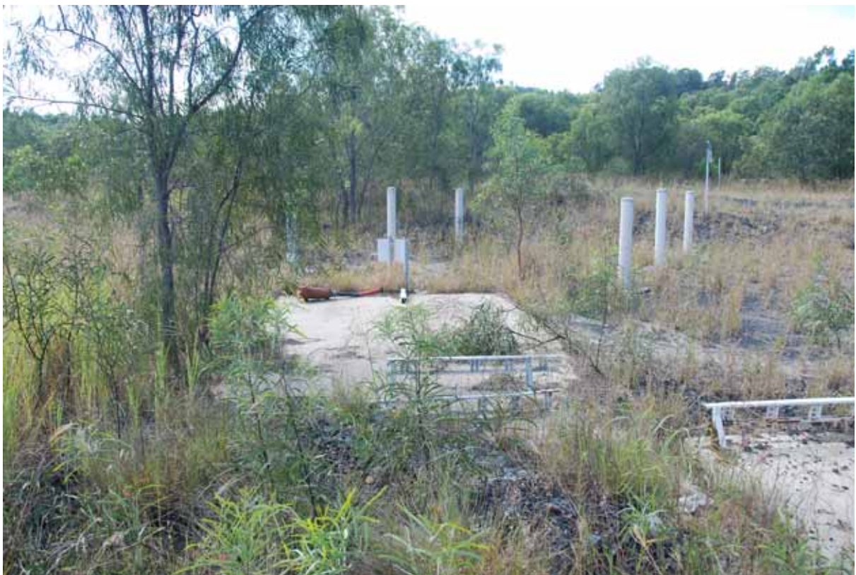
B5 – Concrete Steel Pole
