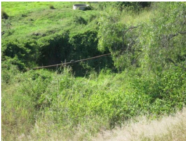
Figure 2.11 Washed out rail bridge
