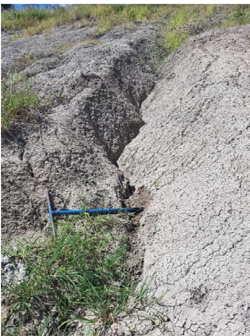
Plate 3 Gully erosion within Area A
