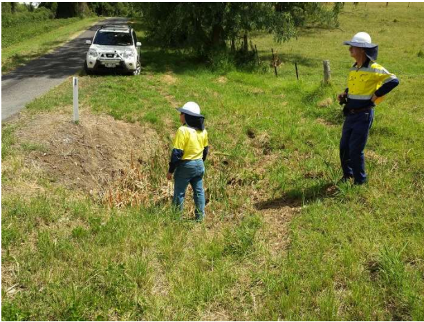
Figure 2.6 Silted up culvert on Blakes Road
