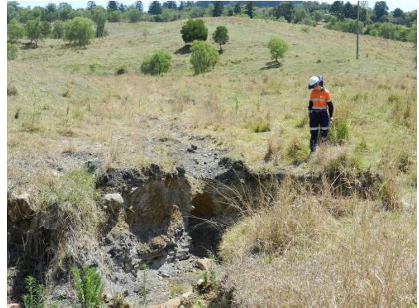
Figure 2.3 Headcut advancing upstream into fill
