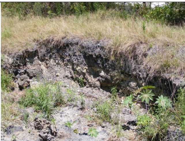
Figure 2 Runoff from the access road, flowing into unconsolidated waste material, has caused a significant gully.
