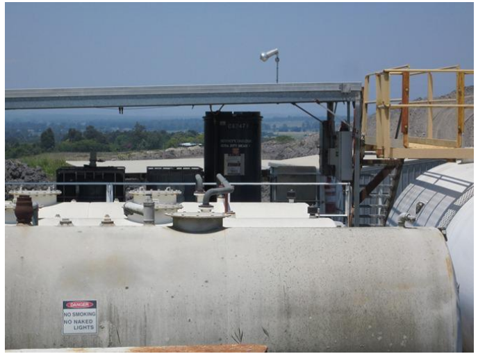
Photograph 8 – Zoomed in shot of fuel farm showing other fuel storage under roofing (15/11/11).
