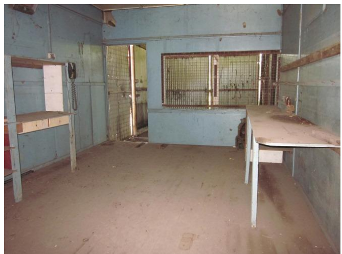
Photograph 52 – Inside the old house with walls constructed of potential asbestos containing materials (15/11/11).
