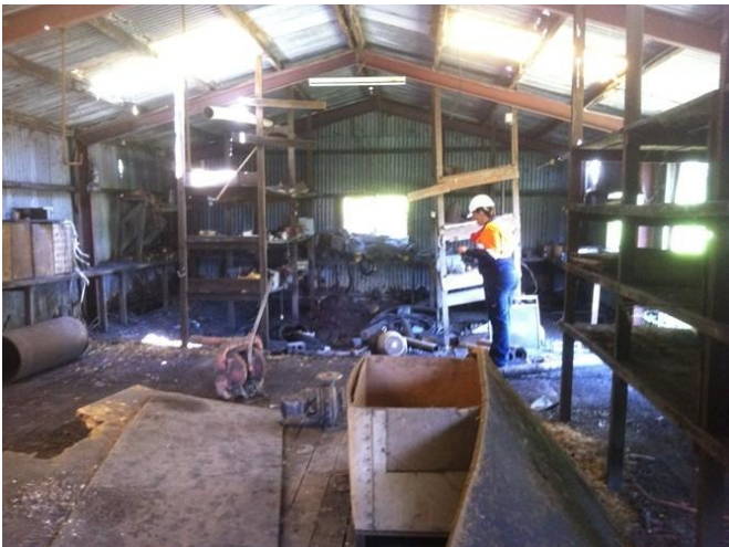
Photograph 85 – Spare parts and storage shed from underground era, wooden floors collapsing (15/11/11).
