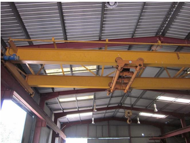
Photograph 63 – Overhead gantry crane in the large workshop building, known as the Operations workshop (15/11/11).
