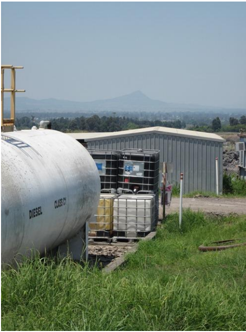
Photograph 19 – Zoomed in shot of the fuel storages in the fuel farm area, with views to the south of the site (15/11/11).
