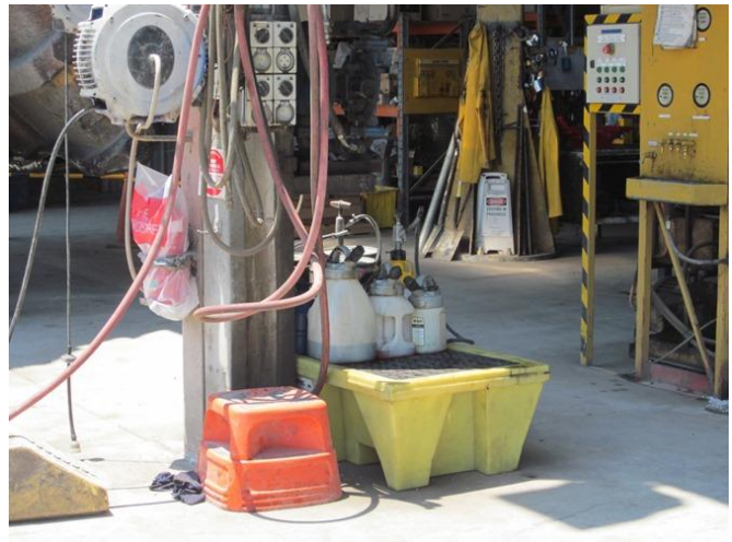
Photograph 22 – Small volumes of chemicals stored in proximity to the servicing area, observed relatively clean floors (15/11/11).
