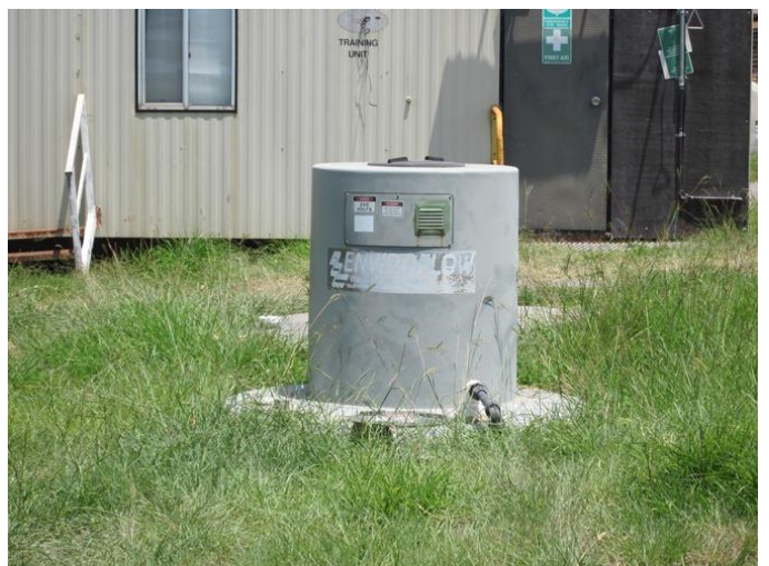
Photograph 6 – Septic tank system for office and workshop buildings facilities (15/11/11).
