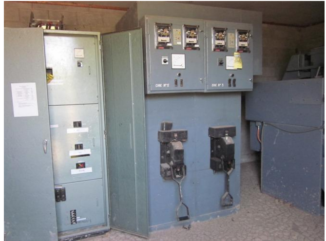
Photograph 48 – Old electrical equipment now decommissioned (15/11/11).
