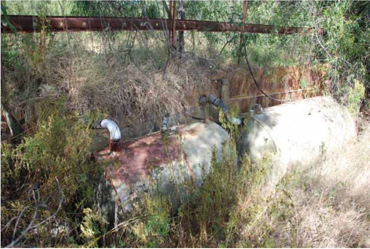
B9 Steel Tank
