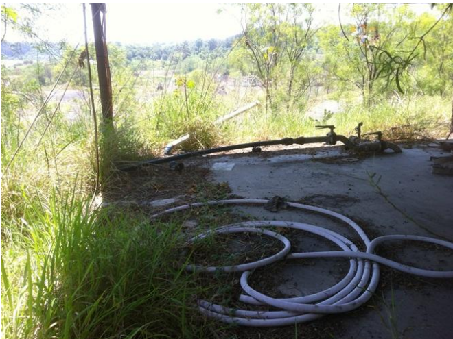
Photograph 79 – Pipe work and hosing related to the fire fighting water supply onsite (15/11/11).
