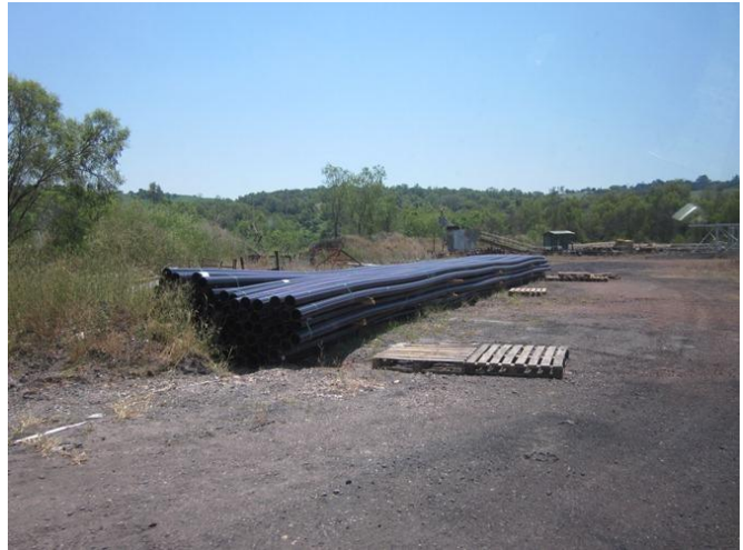
Photograph 32 – Storage of materials in the laydown area adjacent to the eastern site entrance (15/11/11).
