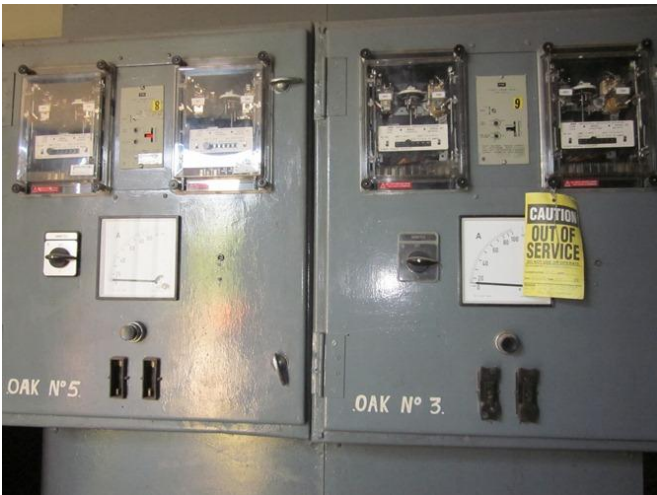
Photograph 49 – Electrical power mains for the previous underground tunnel workings (Oakleigh No. 3 and No. 5) (15/11/11).
