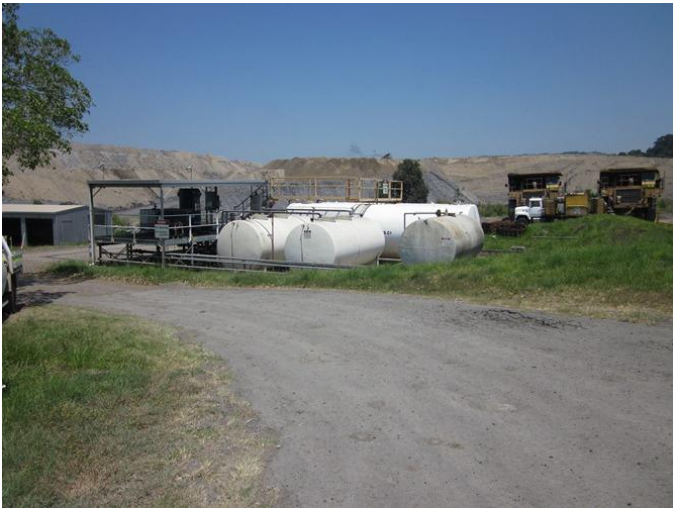
Photograph 7 – West Pit fuel farm with 5 above ground storage tanks observed (15/11/11).
