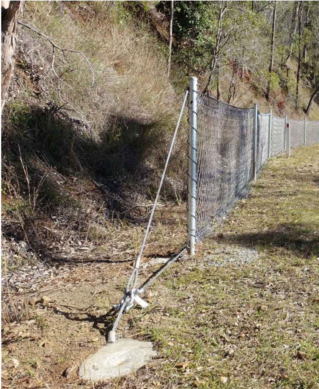
Figure 30. Example of a 1.5m high, 10 kJ capacity, proprietary rockfall barrier. This style of barrier can have a 100 year design life.
