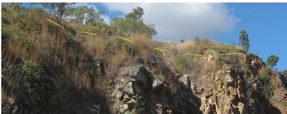
Figure 7. Highlighted is the base of the shallow cover of soil above moderately- to highly-weathered limestone midway along the east wall. Vegetation density is high behind the crest.
