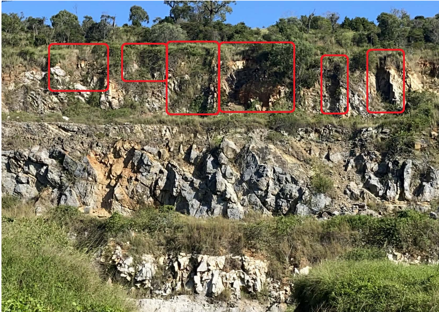
Figure 28. Examples of locations along the crest of the west wall where detachment of masses of rocks of bench scale resulted in the crest breaking back by up to 8.5 m.
