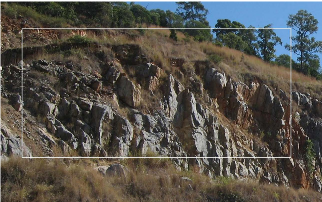
Figure 11. Weathering of clay infill within karst has contributed to the irregular sawtooth surface below the crest at the north end of the west wall.
