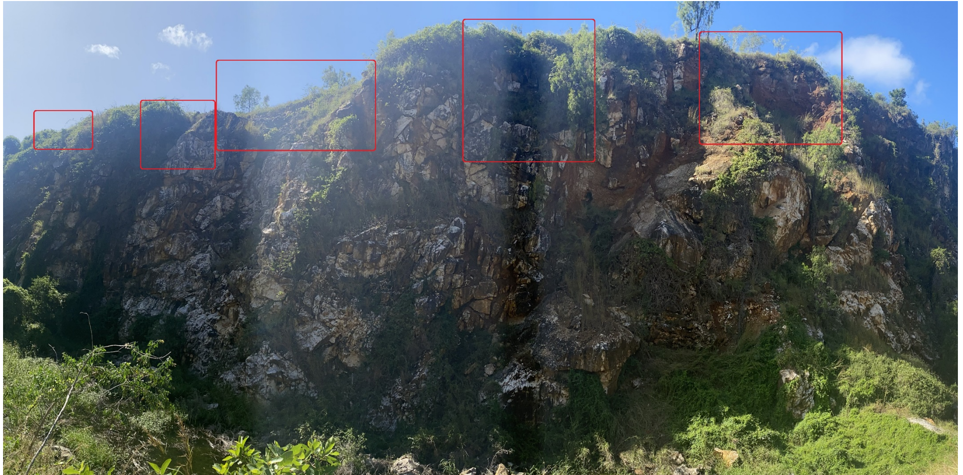
Figure 27. Example of locations along the crest of the east wall where detachments of rocks of inter-ramp and overall scales resulted in the crest breaking back by up to 6.3 m.
