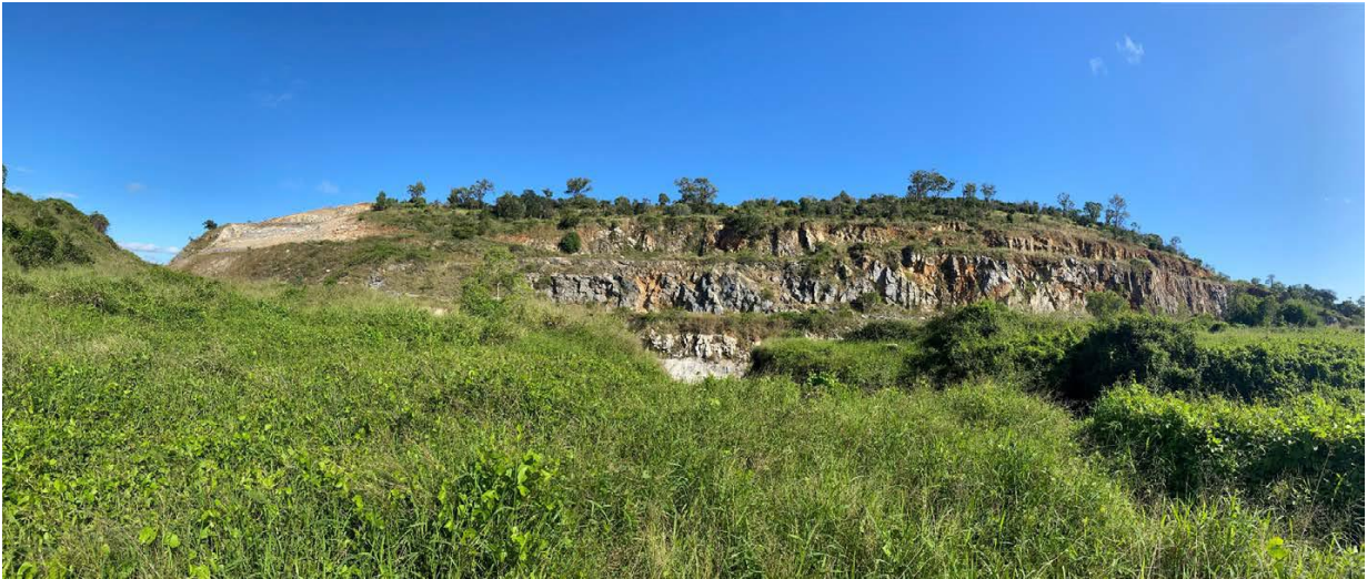
Figure 23: Good vegetation in disturbance areas at the crest of the west wall of void at the Marmor Operations with groundcover, shrub and tree establishment on benches and good groundcover establishment in areas reworked in 2014 to the left
