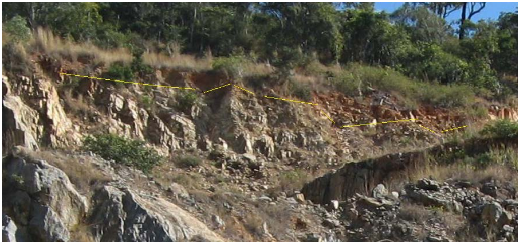
Figure 6. Highlighted is the base of the shallow cover of soil above highly- to extremely-weathered limestone at the north end of the west wall. Vegetation density is high behind the crest.
