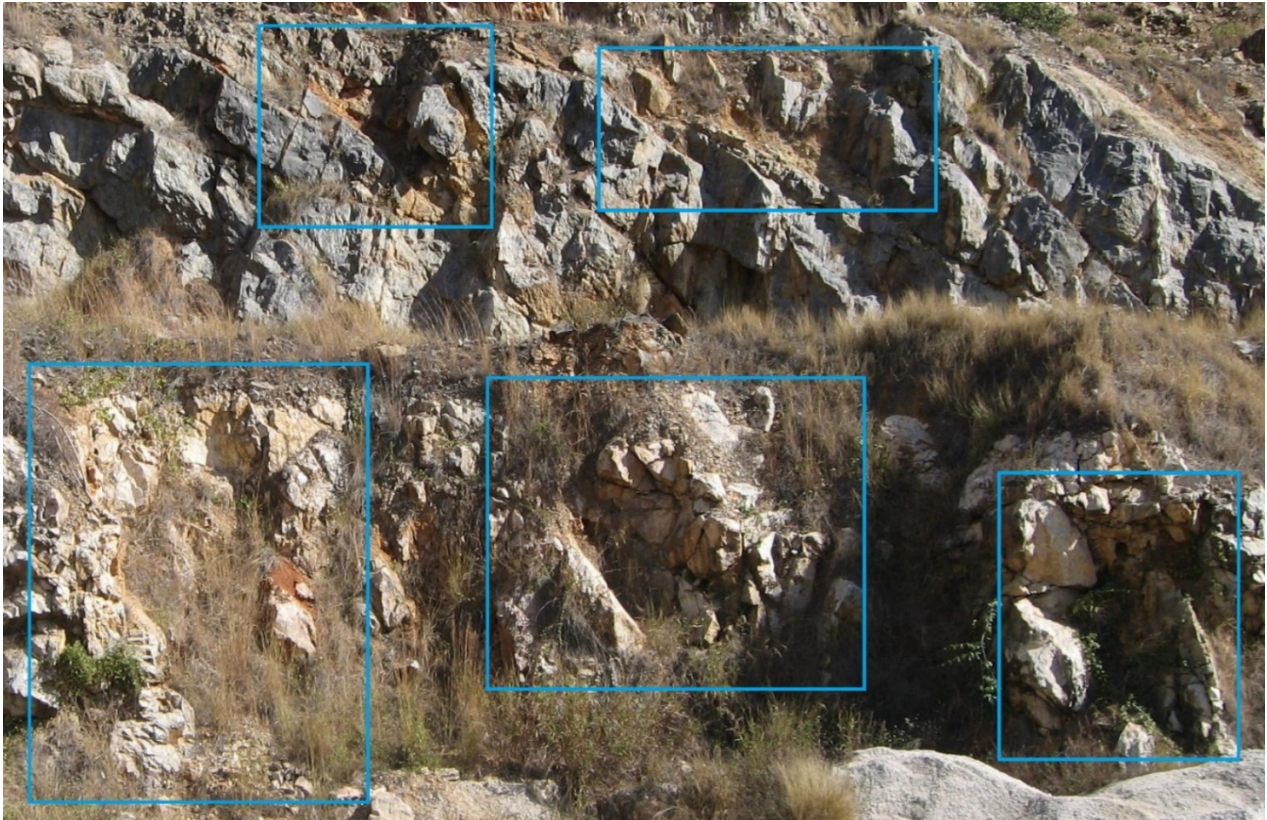
Figure 25. Highlighted at the north end of the west wall are examples of bench scale masses of rocks that have detached by toppling from, and sliding along, one or two discontinuities, predominantly from Sets 3, 5 and 7. Multibench (i.e., inter-ramp) scale instabilities have not occurred on this wall.
