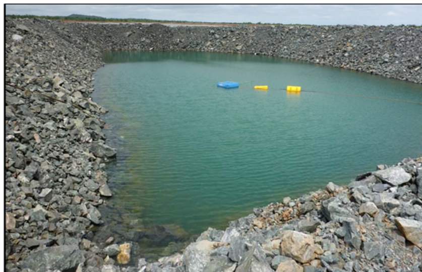
Figure 7-2 – Rock ring with submersible decant pumps
