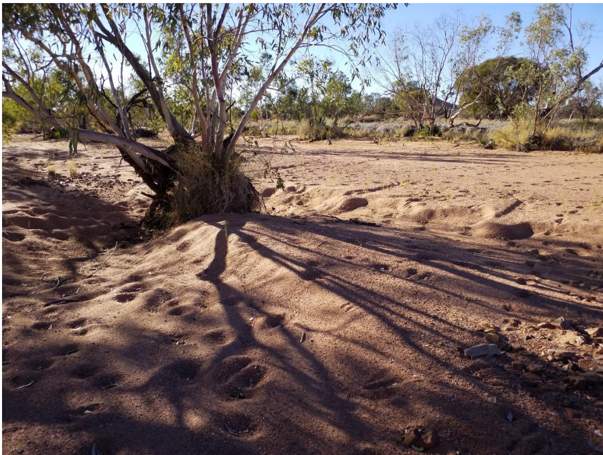
Figure 3: Washout around existing tree, within creek at water storage facility.
