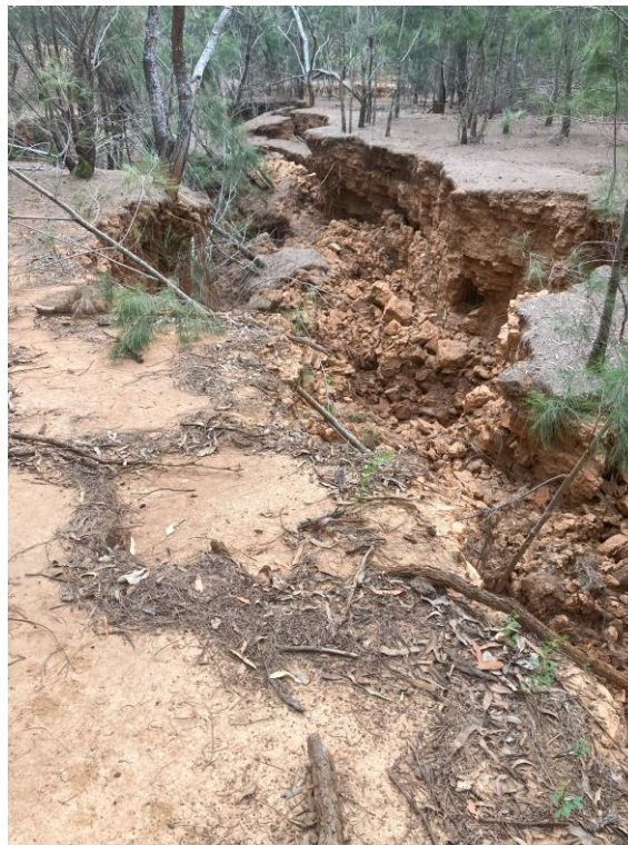
Figure 31: Head cut on Basin 1 Gully 4 – April 2023
