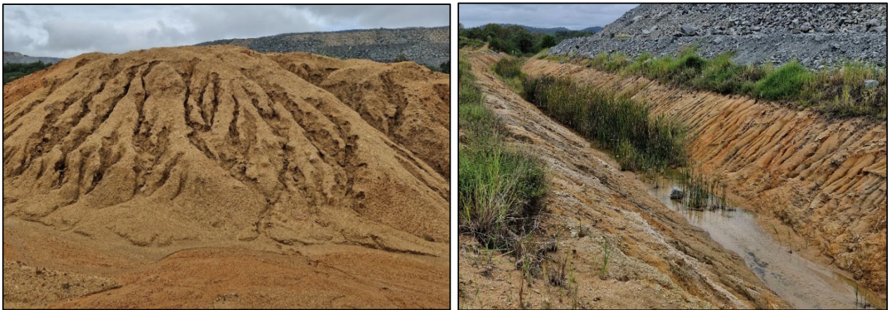
Figure 4.3: Rill erosion on sloped soil material to the north of the TSF.
