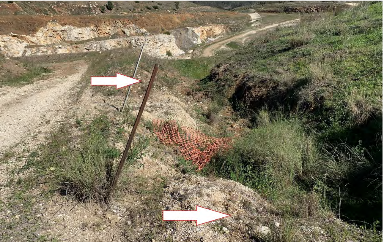
Figure 37. Gully cut by water shedding off the central ramp on the north wall of the East-West pit requires lining and sediment traps.
