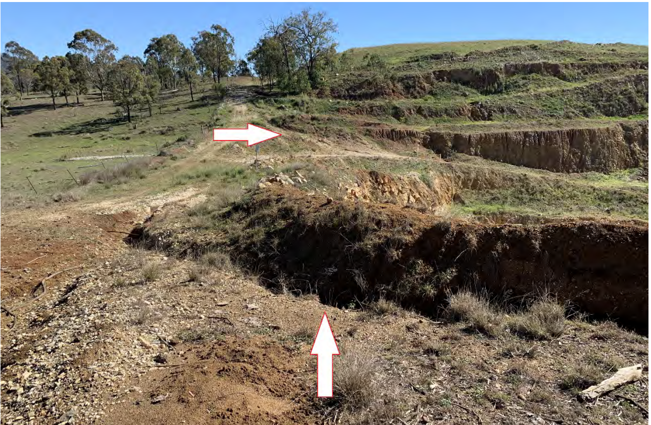
Figure 38. 2 x deep gullies cut by water shedding off the haul-road along the east end of the East-West pit requires repair. Haul-road to be graded to shed water to the east and ripped.
