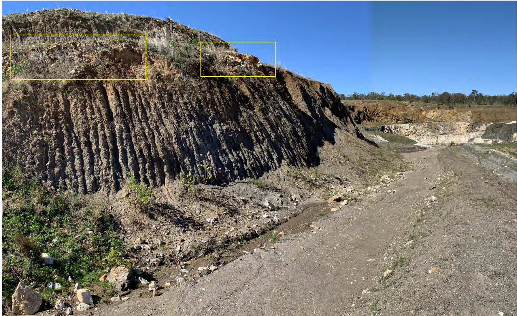
Figure 32. Loose rocks (highlighted) within soil and weathered siltstones near the crest of the batter adjacent to the central ramp in the East-West pit are currently hazards for users of the ramp. Batter should be draped in rockfall mesh, debris removed from the toe and drainage installed across and down the ramp. Flows of water from the overlying 550-mRL berm are not be modified with berm and batter drain and crest bunds.
