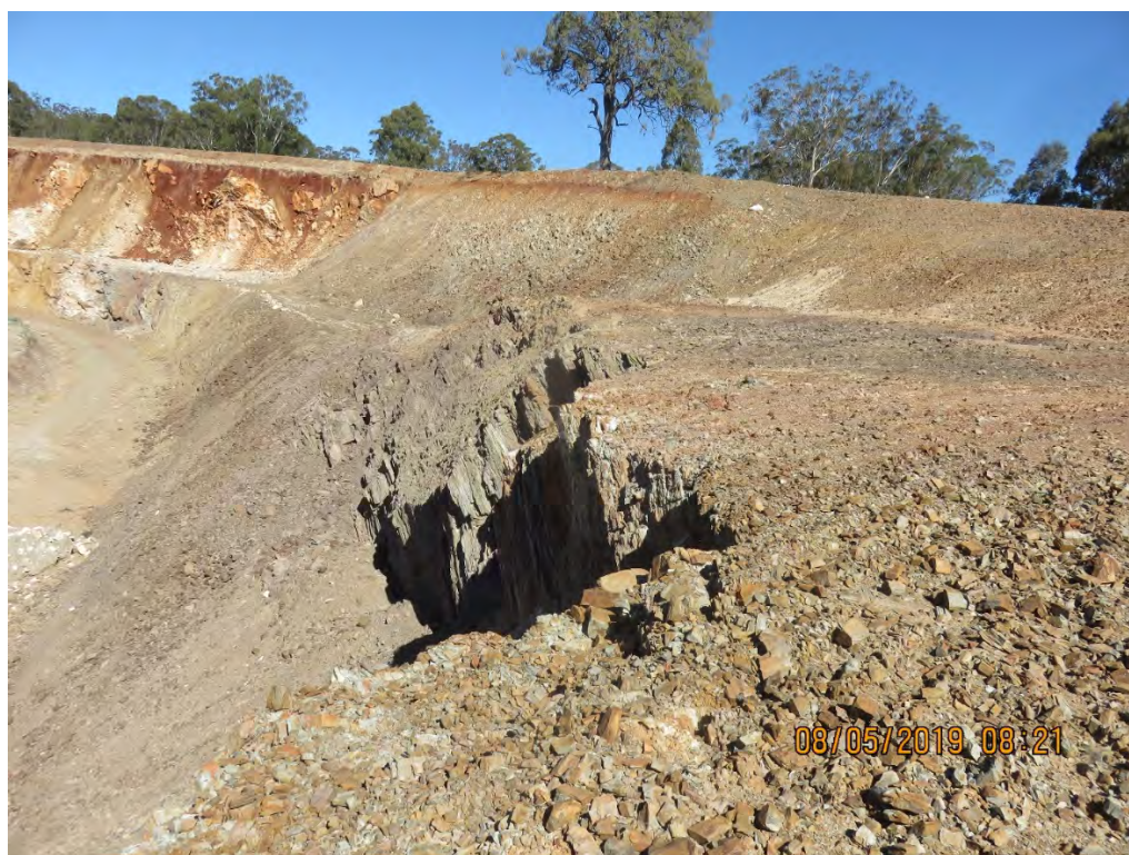
Figure 31. Toppling rocks on an east dipping batter on the upper bench of the Phoenix pit.
