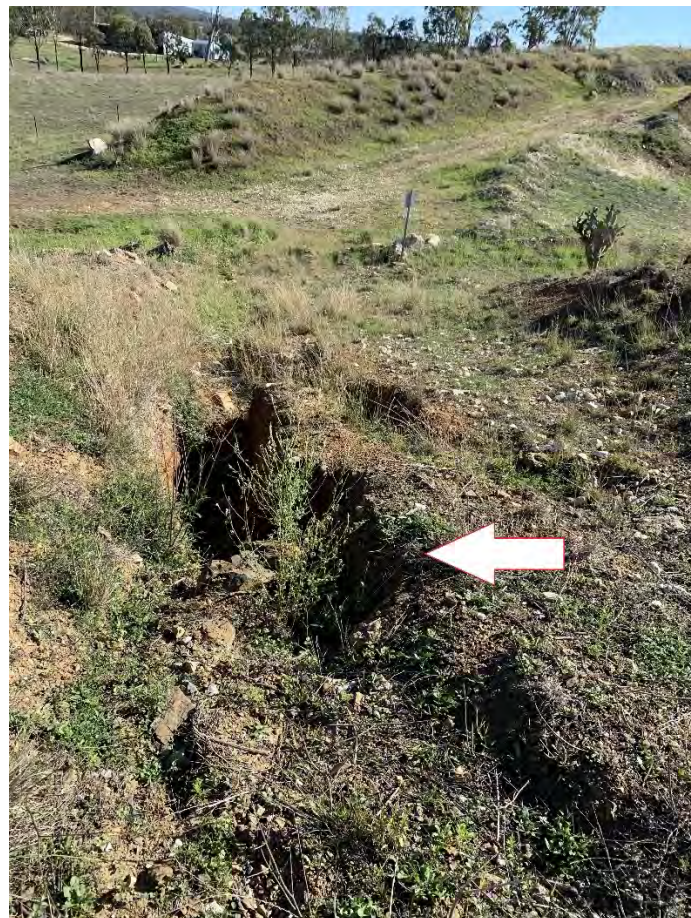
Figure 36. Deep gully cut by water shedding off the west end of WRD 1 is contributing to erosion of the ramp at the west end of the East-West pit. Drain will be remediated when the ramp is removed.
