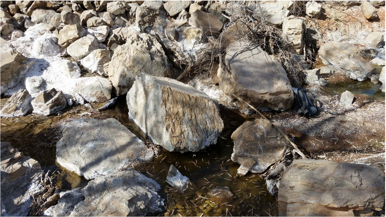
Photograph I-24: TD3 Seepage, Main Seepage Point
