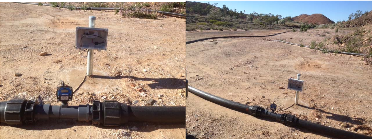
Figure 5-29: BSOC WRD South Seepage transfer pump flow monitoring equipment (July, 2016)
