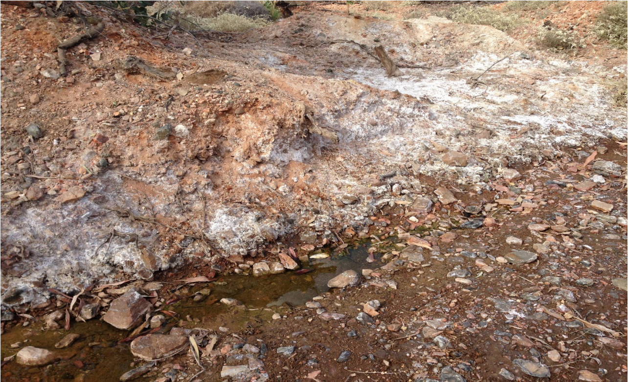
Photograph I-22: Seepage in Diversion Drain, Upstream of TD3 Seepage, Facing South
