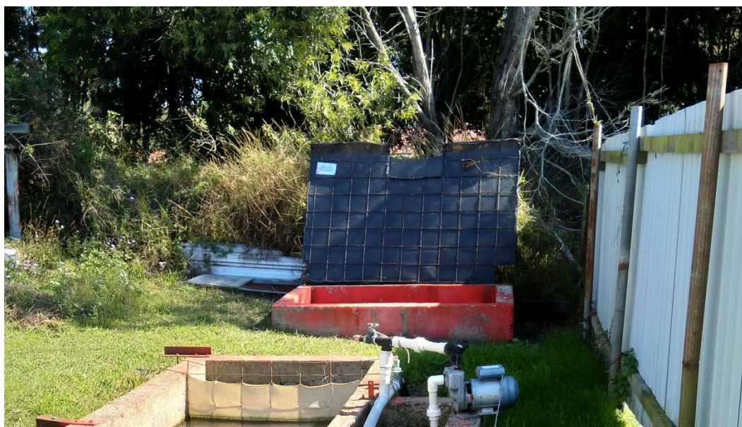
Figure 19: Chlorine Contact Tank
