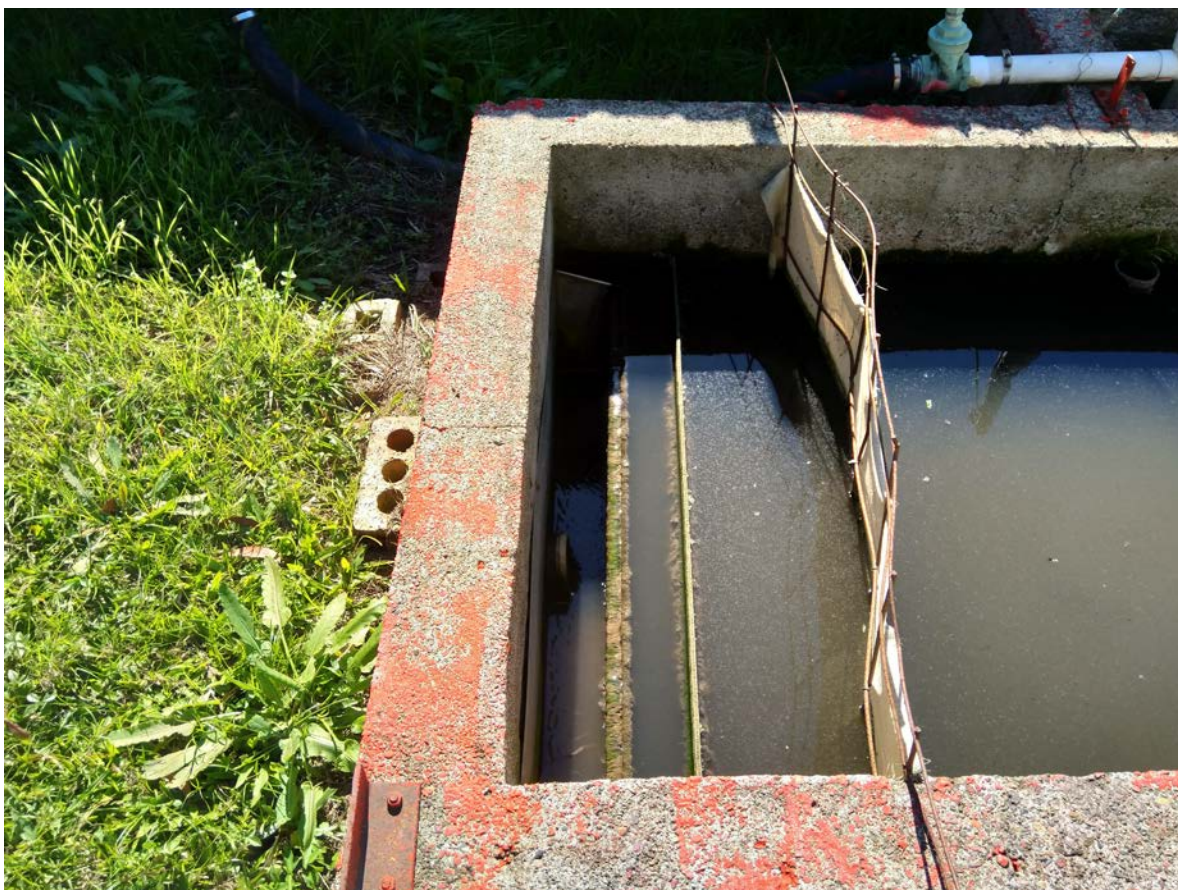
Figure 18: Effluent Weir and scum baffling
