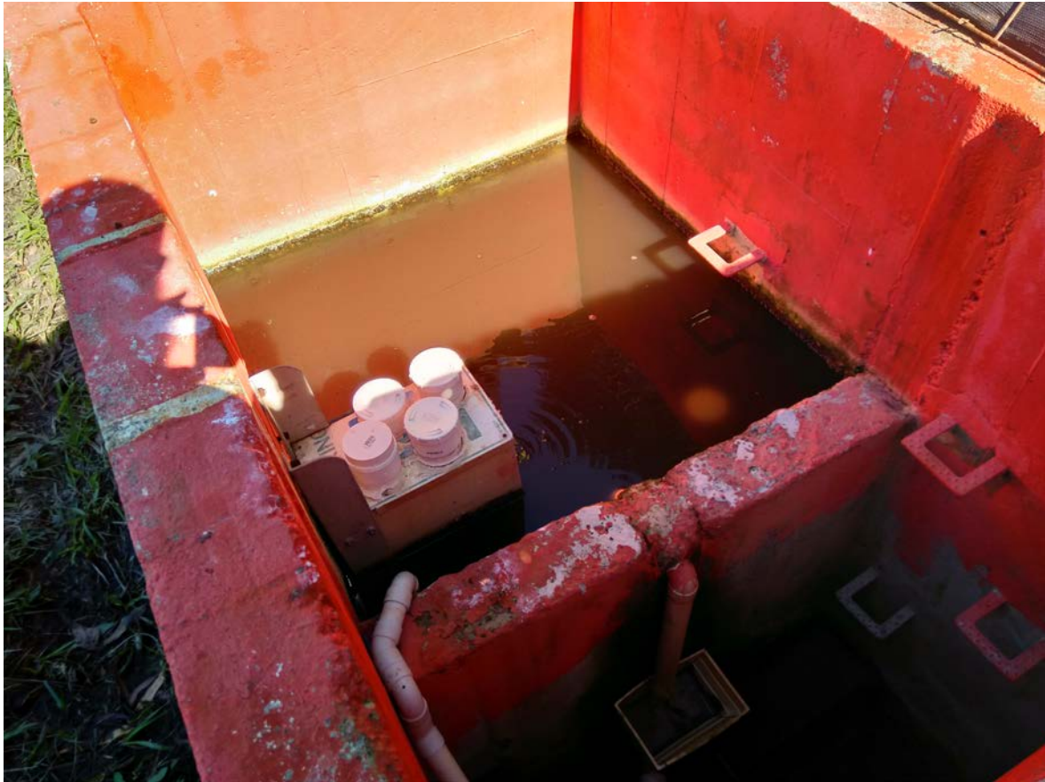
Figure 20: Contact Chamber and Chlorinator
