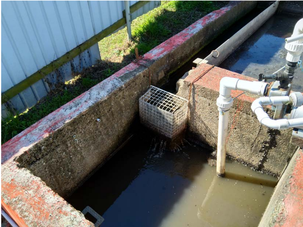
Figure 9: Clarifier Discharge Basket and trickling filter feed pump station
