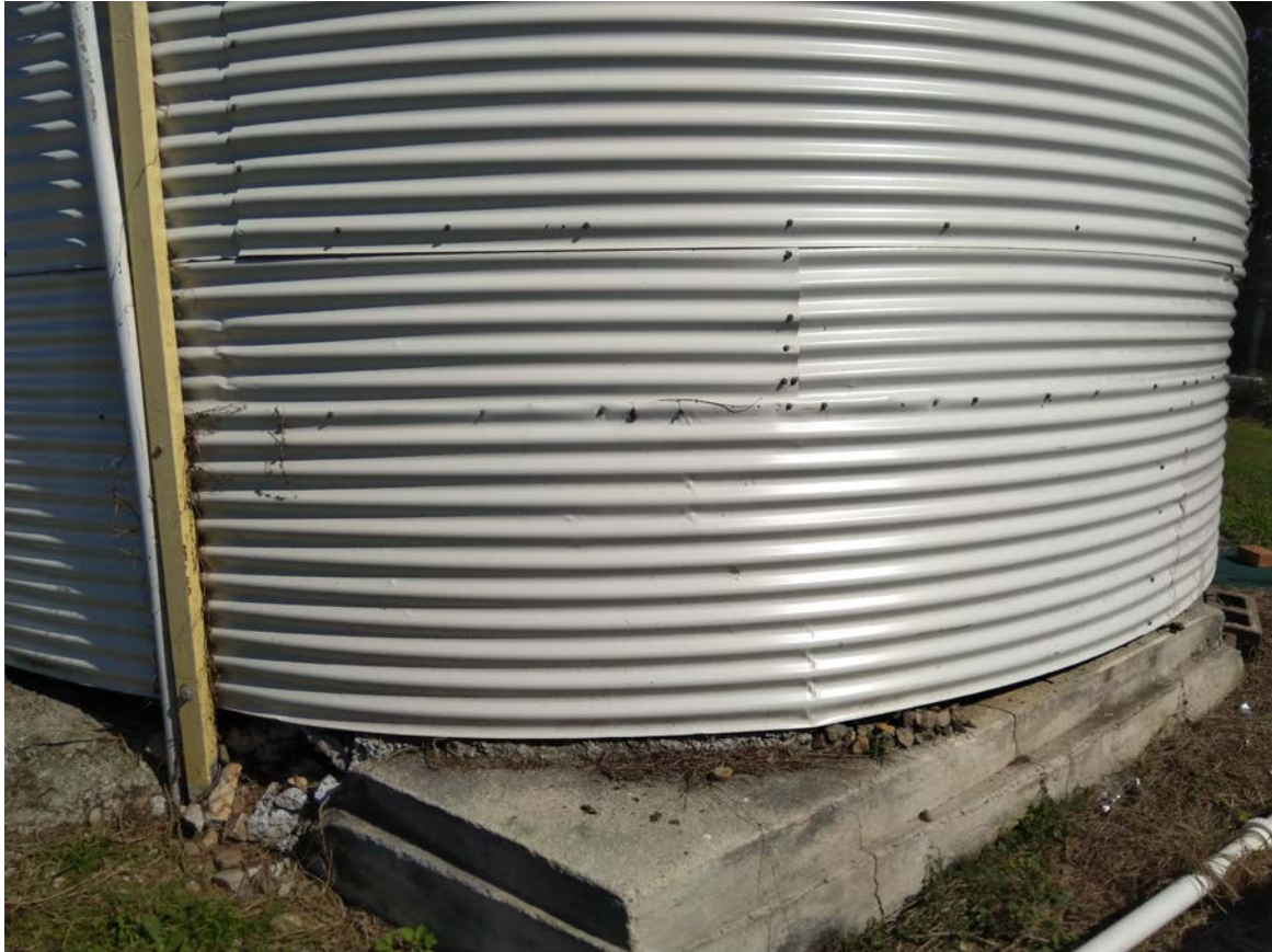
Figure 14: Rock showing at base of unit, slight bulge to exterior corrugated steel wall
