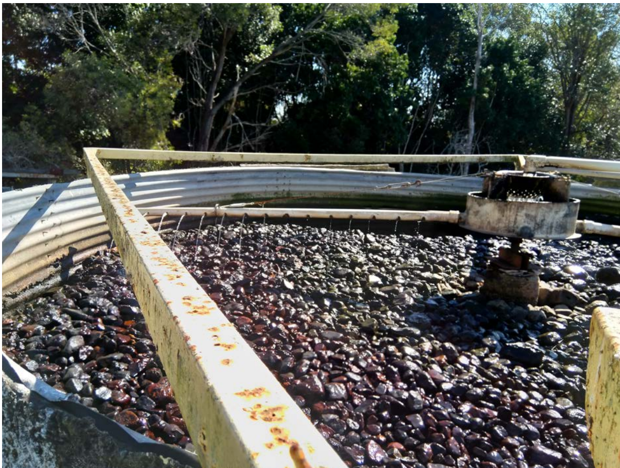
Figure 15: Rotary distributor arm showing poor flow distribution, and significant deflection and significant variance in colour of rock media
