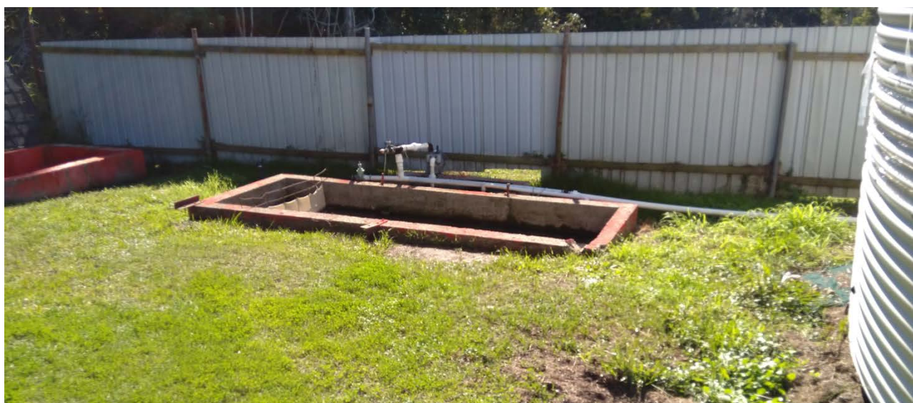
Figure 16: Secondary Clarifier Tank
