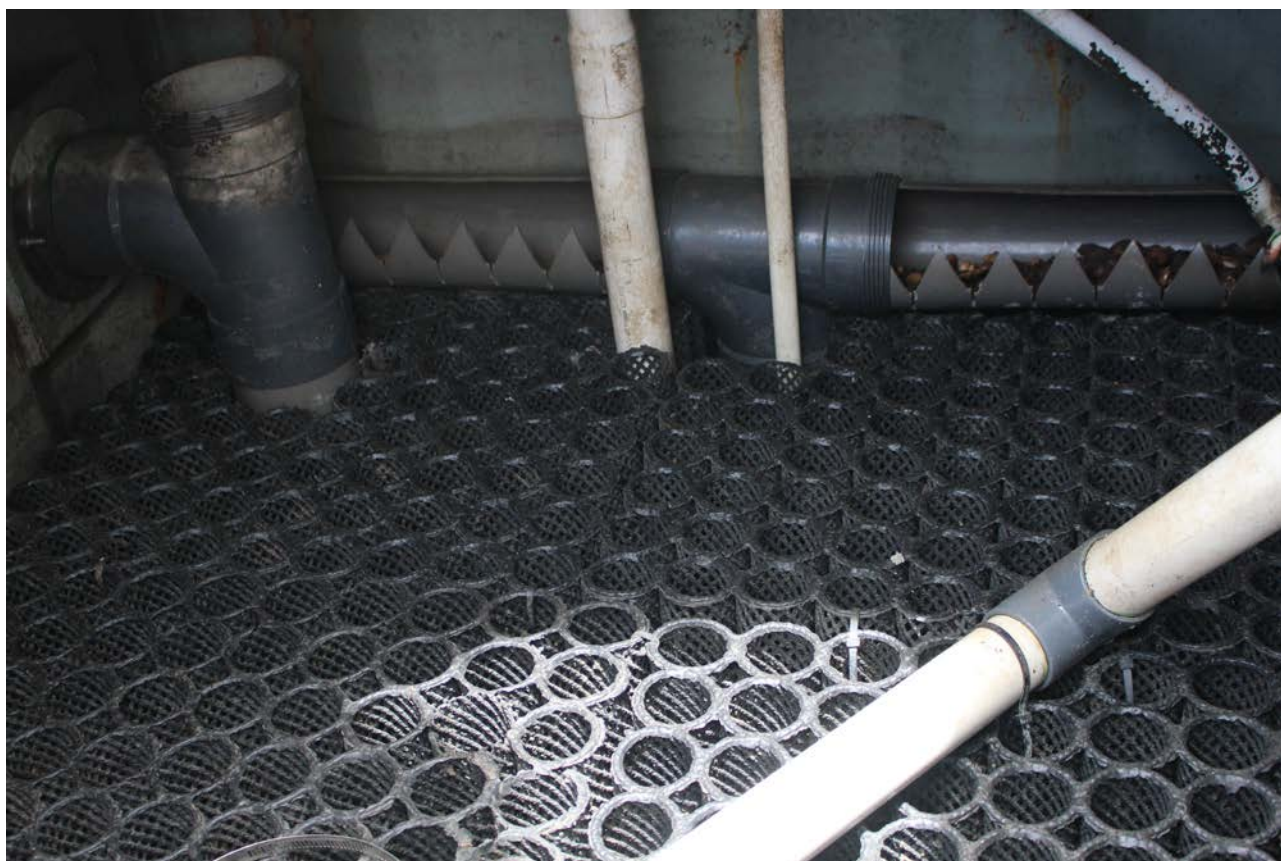
Figure 6: Pre-Anoxic Tank Packing
