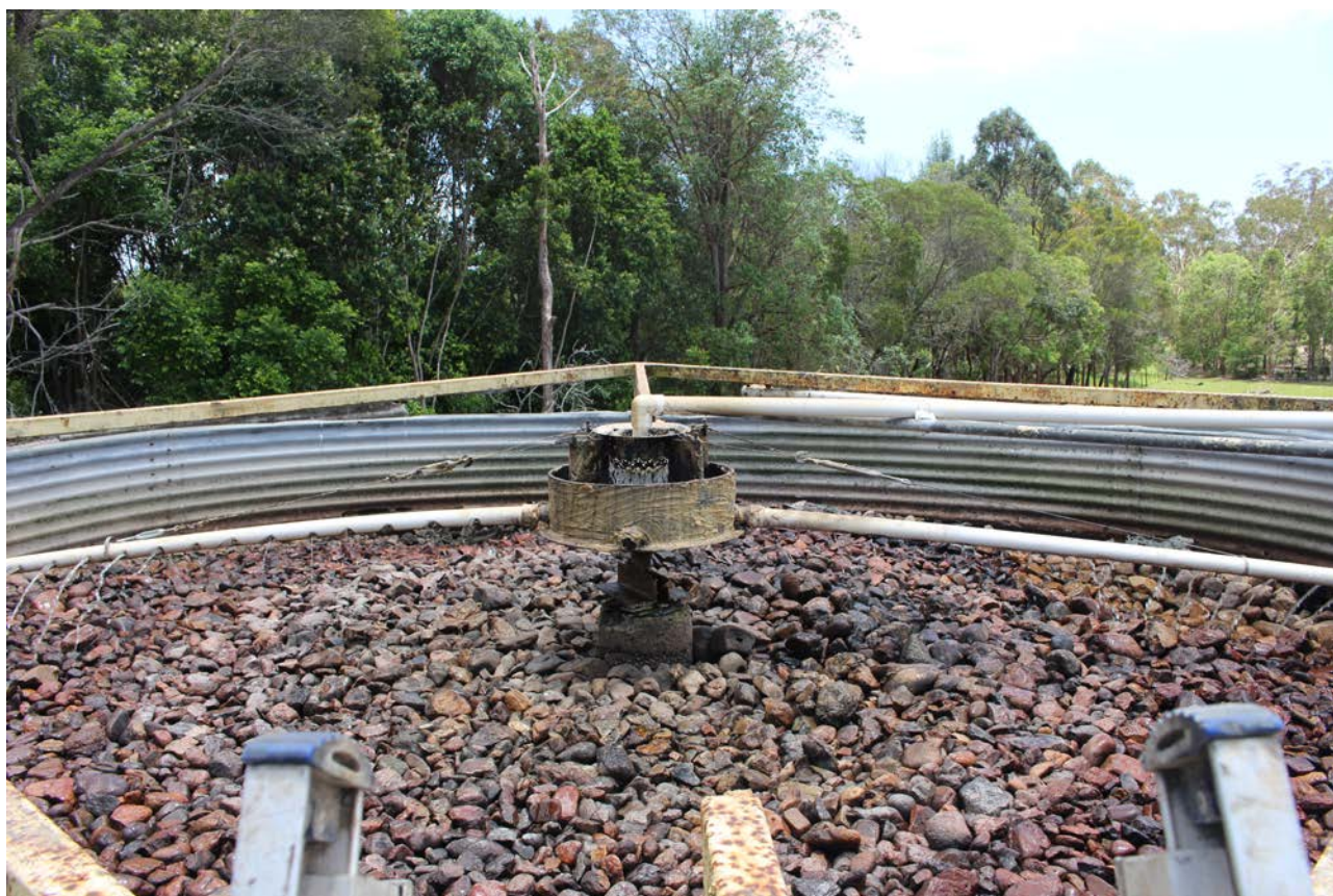
Figure 7: trickling Filter Distributor arm 'sag'
