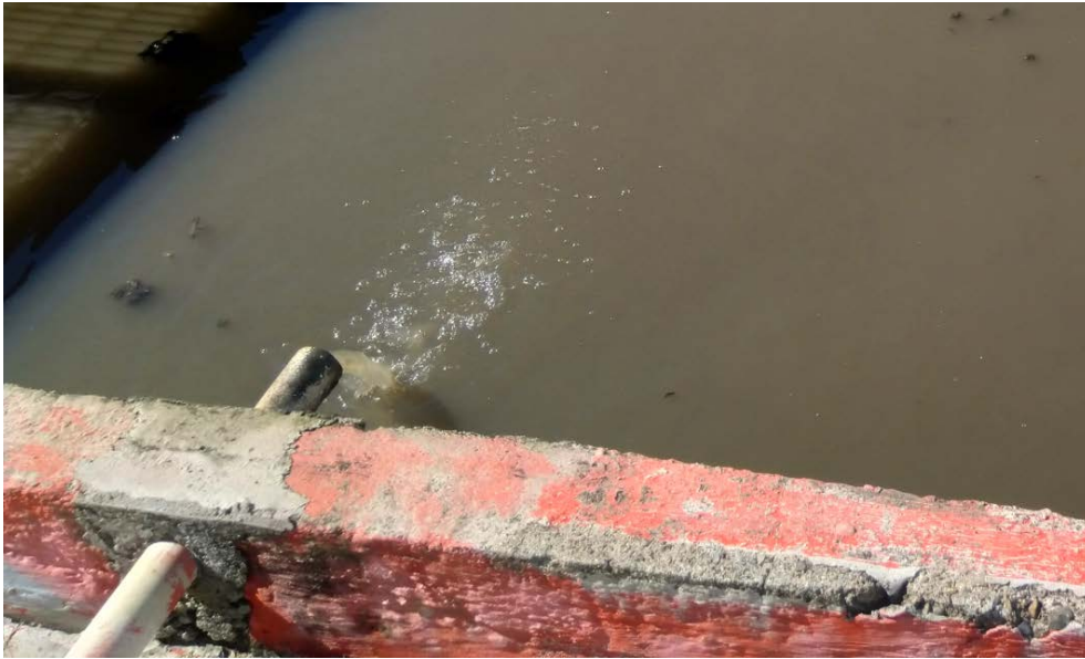
Figure 11 Clarifier RAS/TF Recycle Inlet
