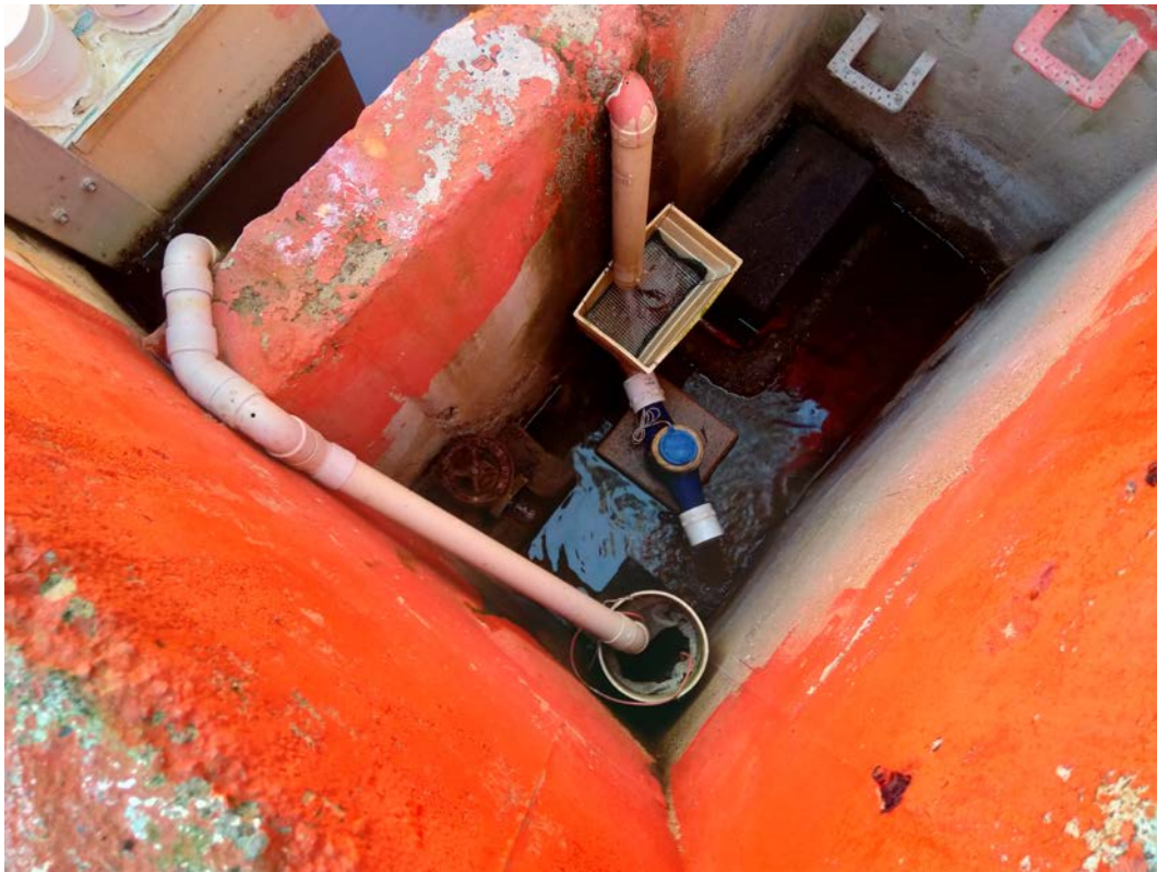
Figure 21: Effluent Discharge Flowmeter
