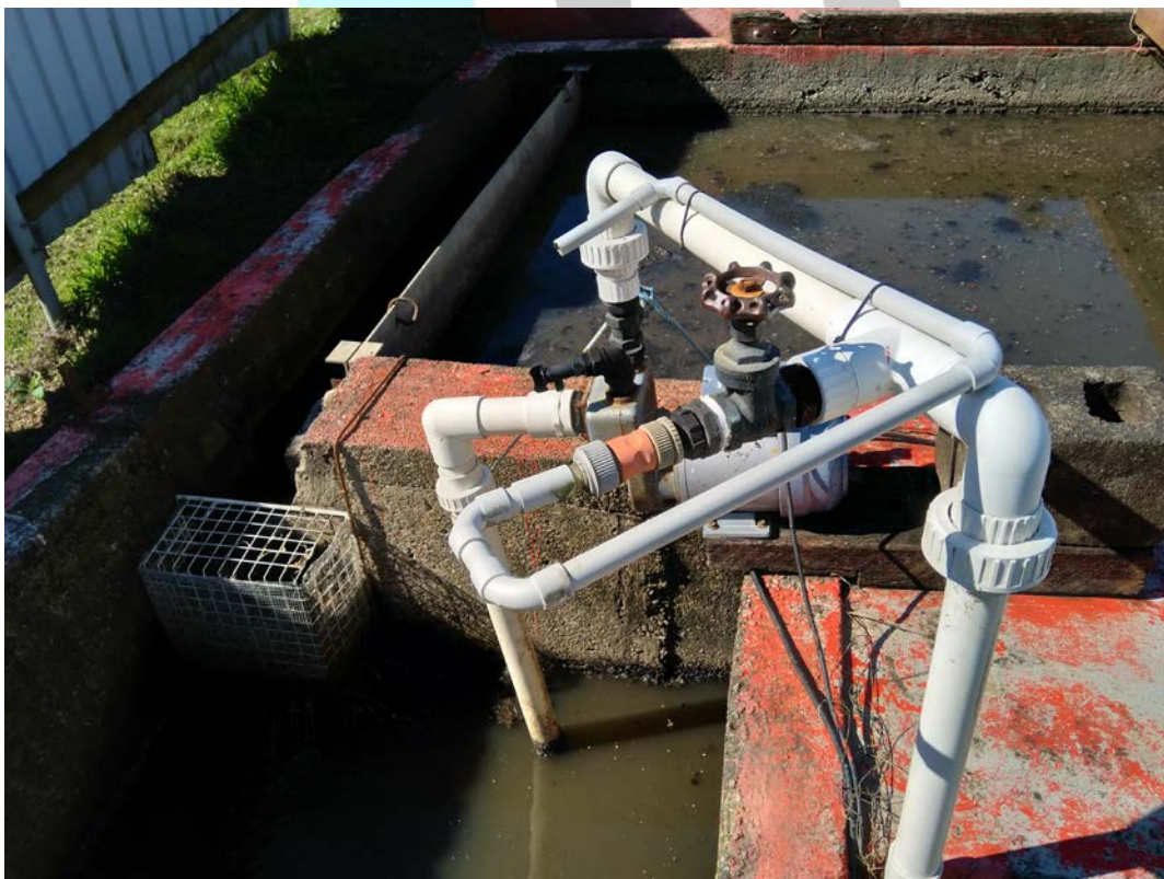
Figure 10: Trickling Filter Feed Pump
