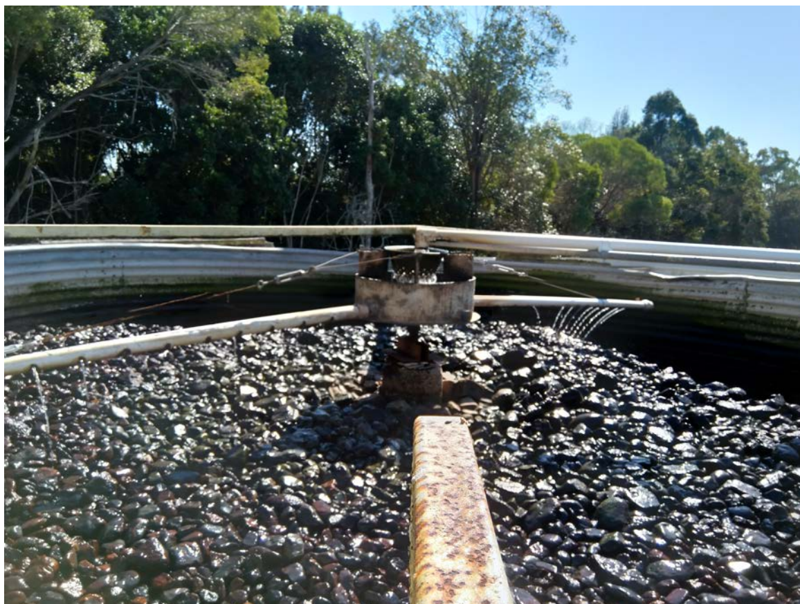
Figure 12: Trickling Filter & Rotary distributor
