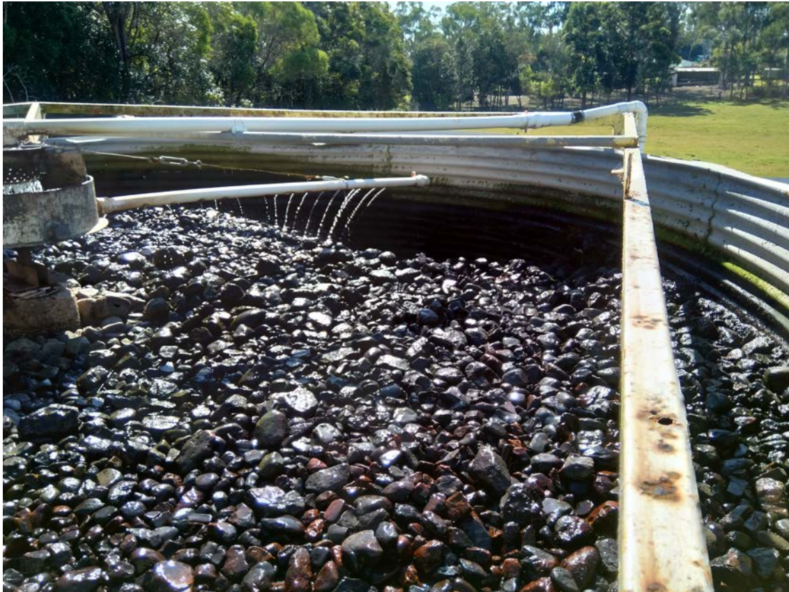
Figure 13: Collapsed Bed Area
