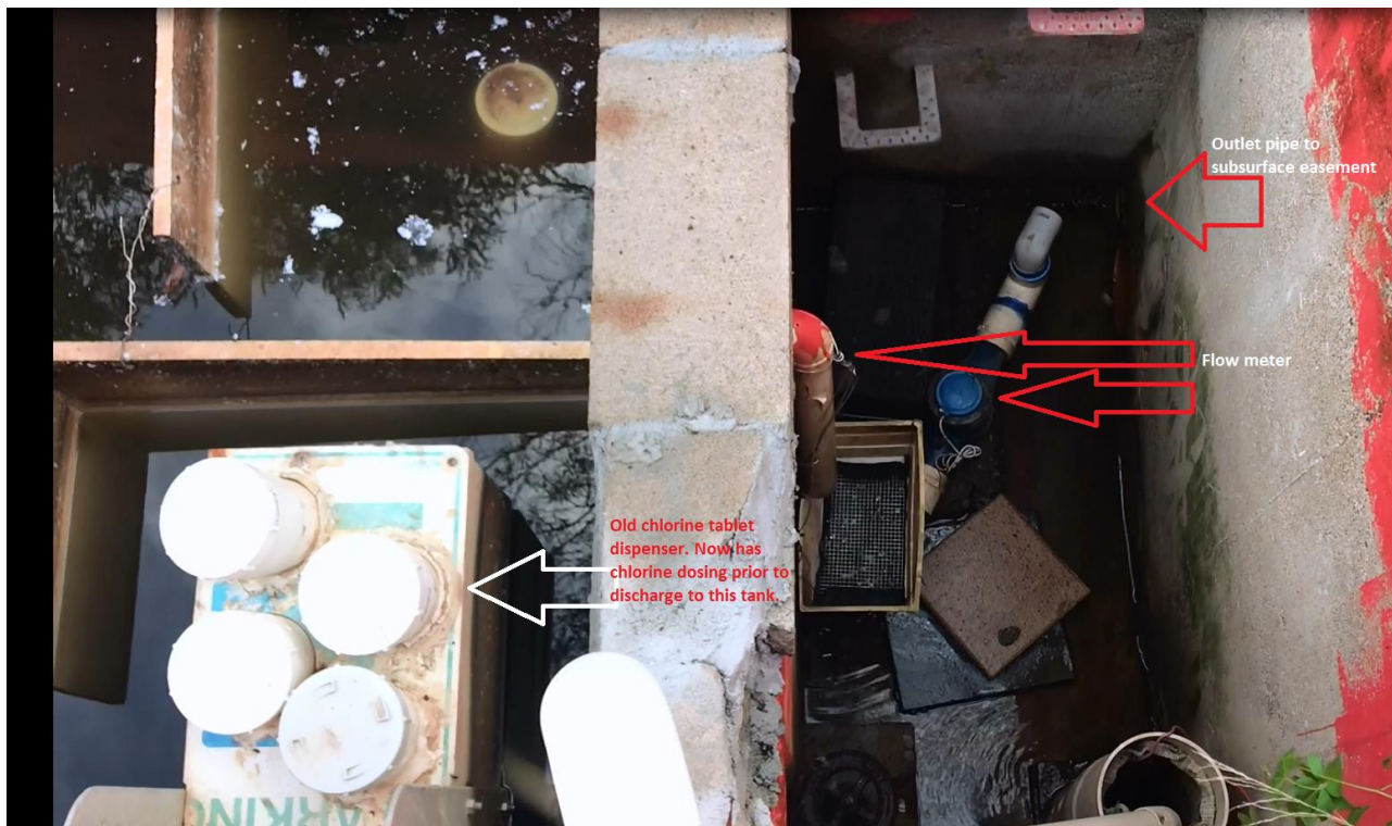
Figure 30 Chlorine contact tank and exit to subsurface drain
