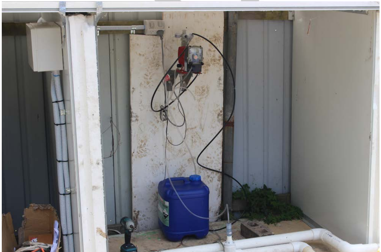
Figure 4: Chemical Metering Pump
