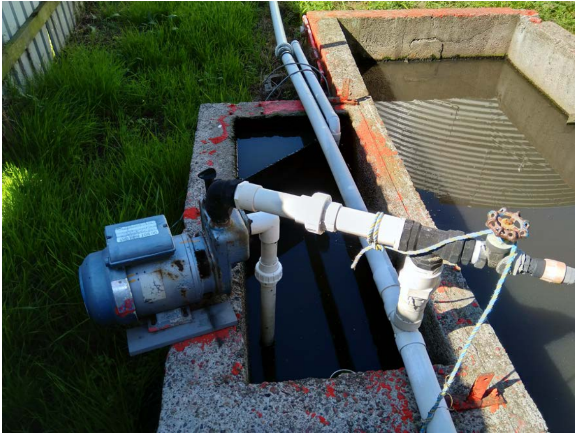
Figure 17: TF Recycle & Return Sludge pumping station
