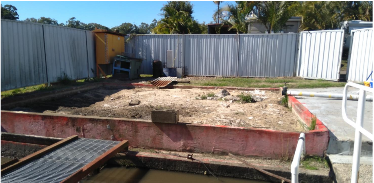
Figure 32 Sludge Drying Bed
