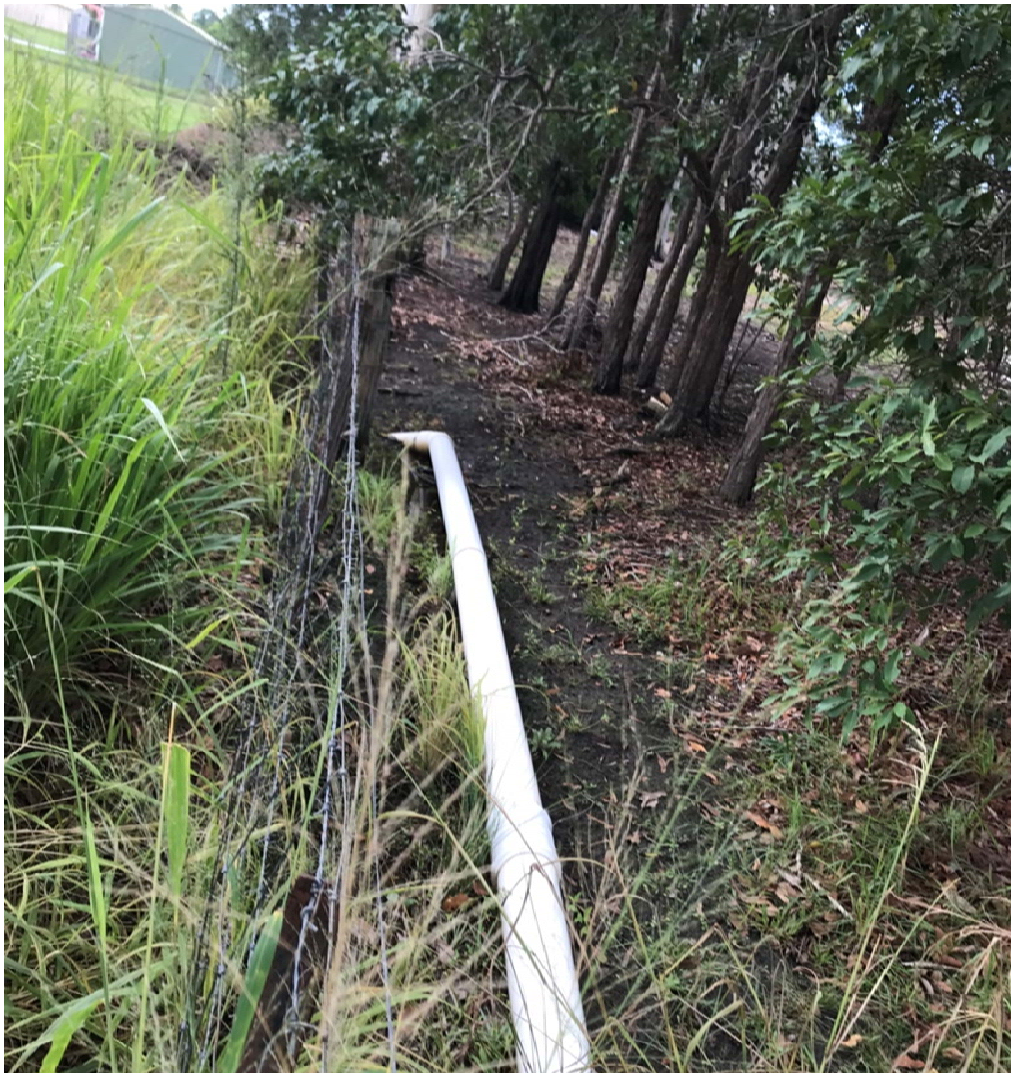
Figure 13: Final effluent discharge pipe near the North West border of lot
