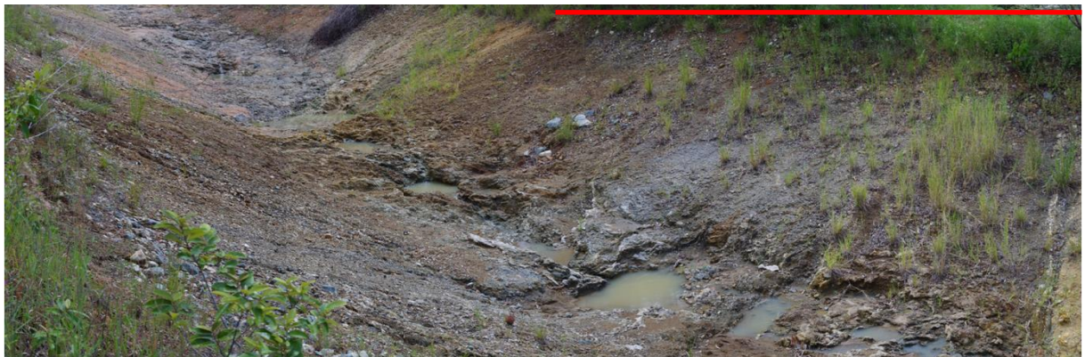
Figure 7: West Dam Fault (marked by red line) exposed in the Western Stormwater Drain 8
