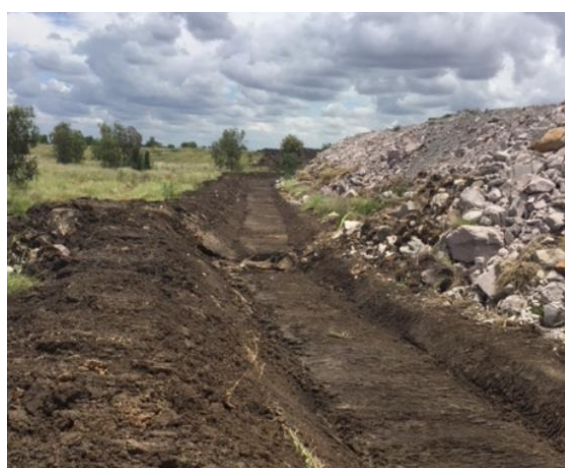
Figure 5.4 Western Drain - on Western Side of Haul Road (Looking North) (22/11/2017)
