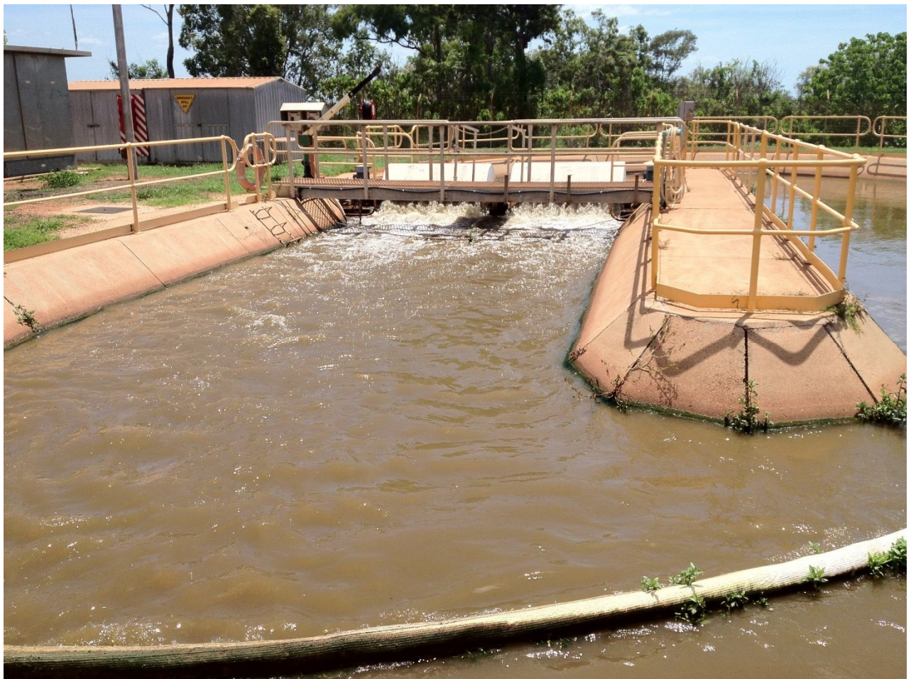
Figure 7: Oxidation Ditch with Brush Aerator at Lorim Point STP, Weipa, Qld
