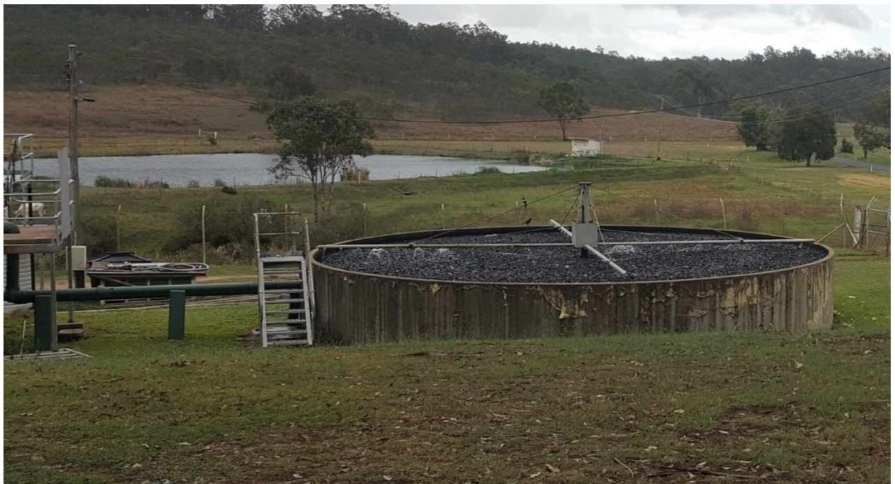
Figure 8: Trickling Filter at Cherbourg STP, Qld
