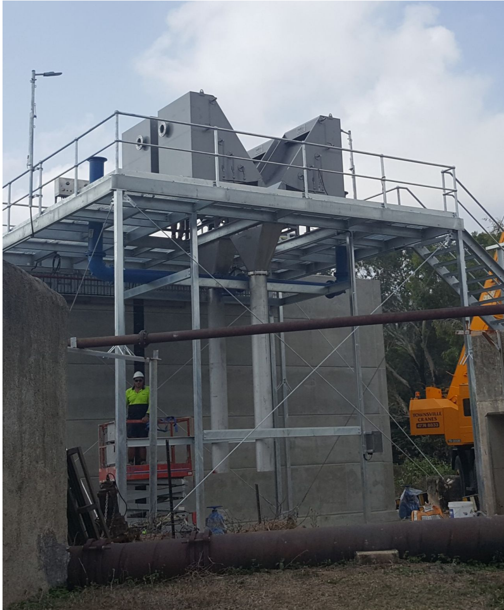
Figure 13 – New Static Rundown Screens at Palm Island. Two screens facing each other is proposed.
