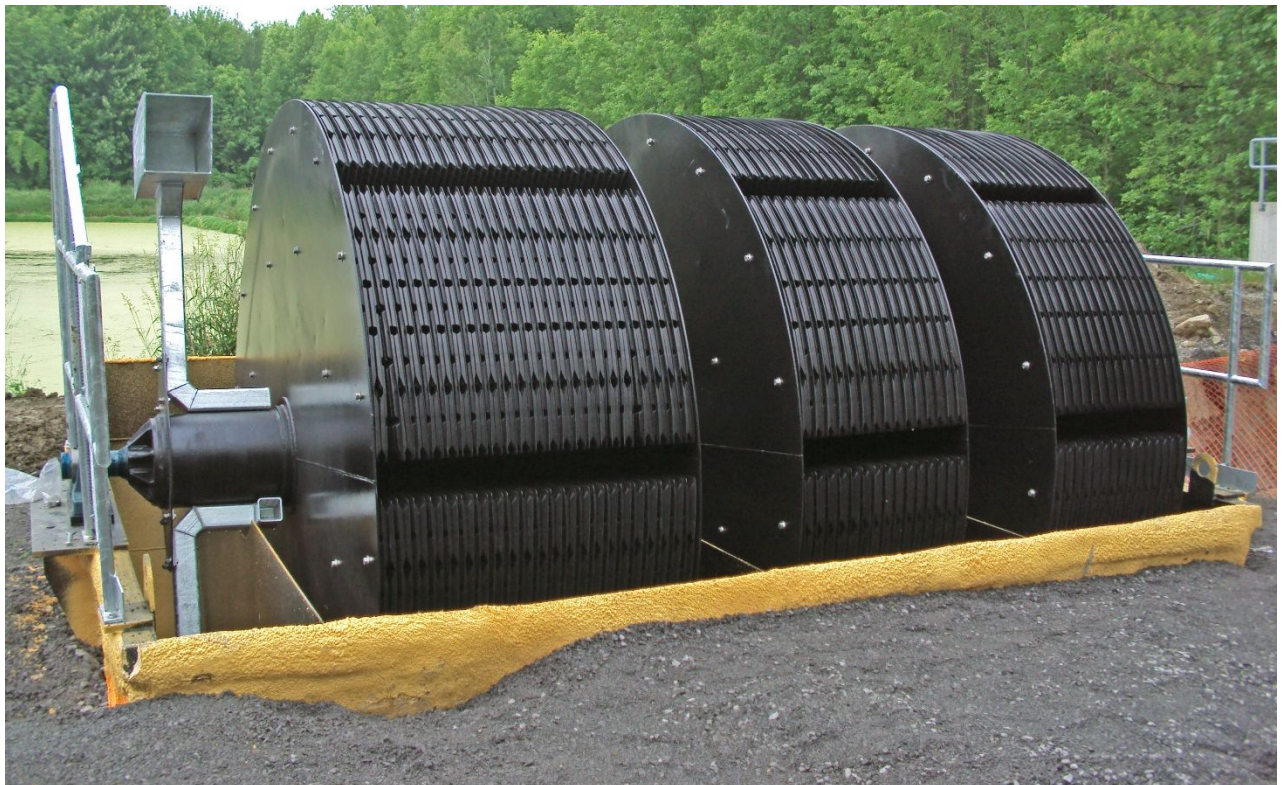
Figure 11: Typical Rotating Biological Contactor
