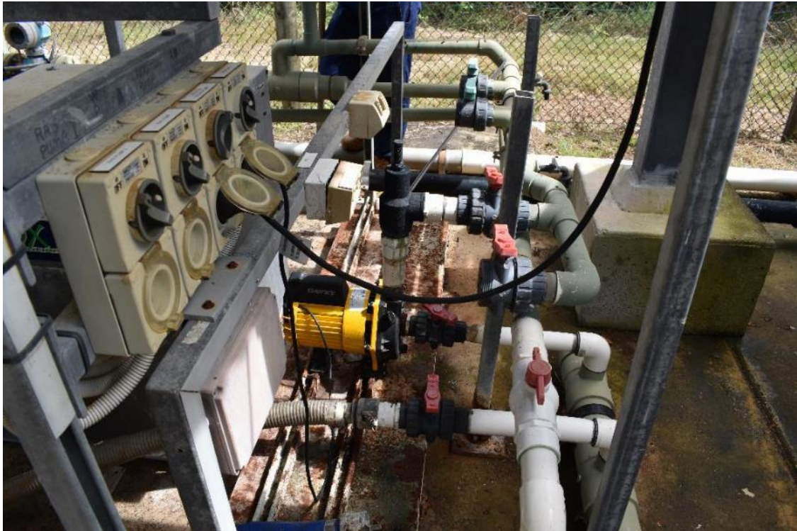
Figure 17 - RAS, WAS & Aerobic Return Pump Station
