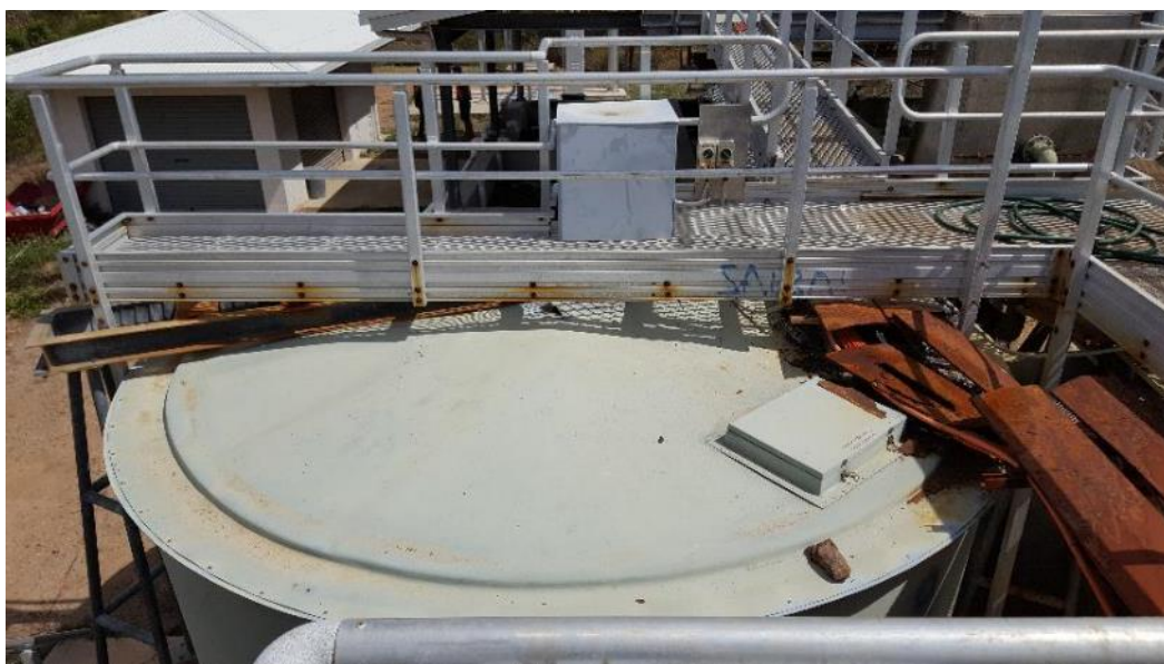
Figure 16 – Anoxic 1 Tank, corroded cable cable trays, fasteners etc.
