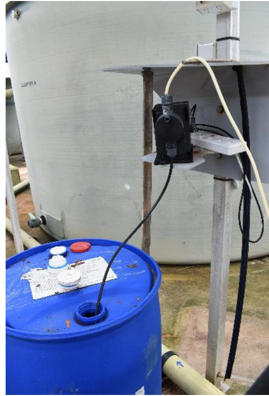
Figure 30 - Sodium Hypochlorite Dosing System
