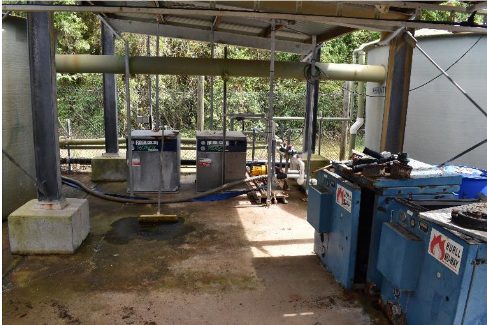
Figure 21 - Aeration blowers (straight ahead) and old blowers (right) had not been removed from site
