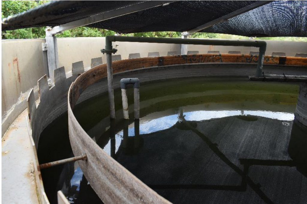
Figure 24 – Clarifier with low level water level and stagnant water
