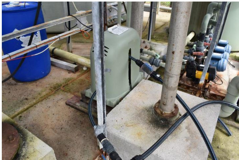
Figure 14 - STP Service Water Booster Pump (Located underneath the clarifier)
