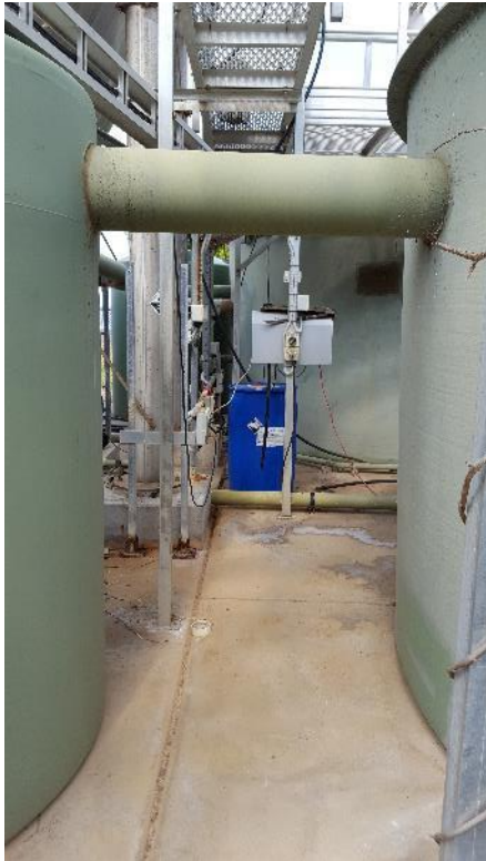
Figure 29 - Sodium Hypochlorite Dosing System
