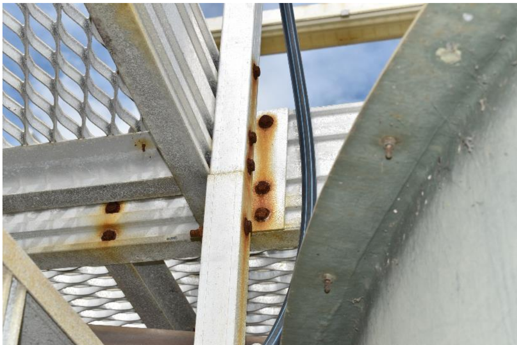
Figure 34 - Corroded Structural Bolts on Platforms
