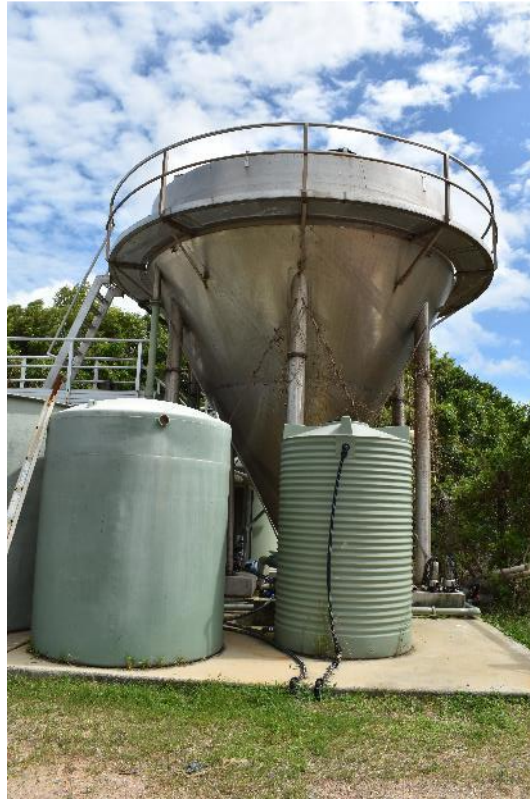
Figure 13 - STP Service Water Tank (Booster set is located under the clarifier)
