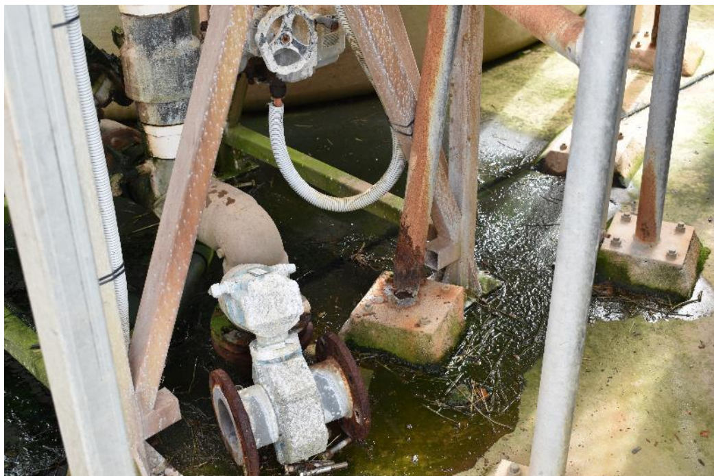
Figure 18 - Corroded mixer supports (typical)
