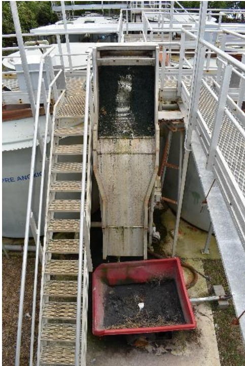
Figure 5 - Static Screen and Screenings Collection Trailer
