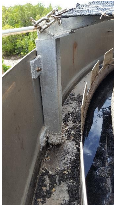
Figure 25 - Corrosion of shade structure supports at connection to Clarifier
