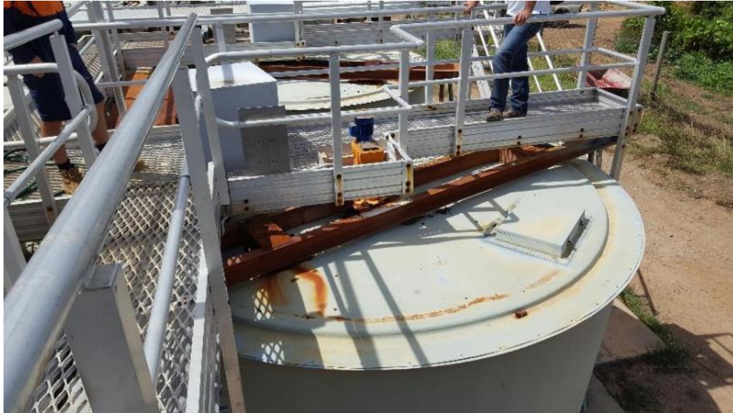
Figure 19 – Corroded Mixer Supports (typical)
