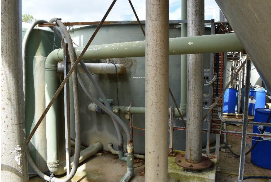
Figure 27 - Chlorine Contact Tank Penetrations
