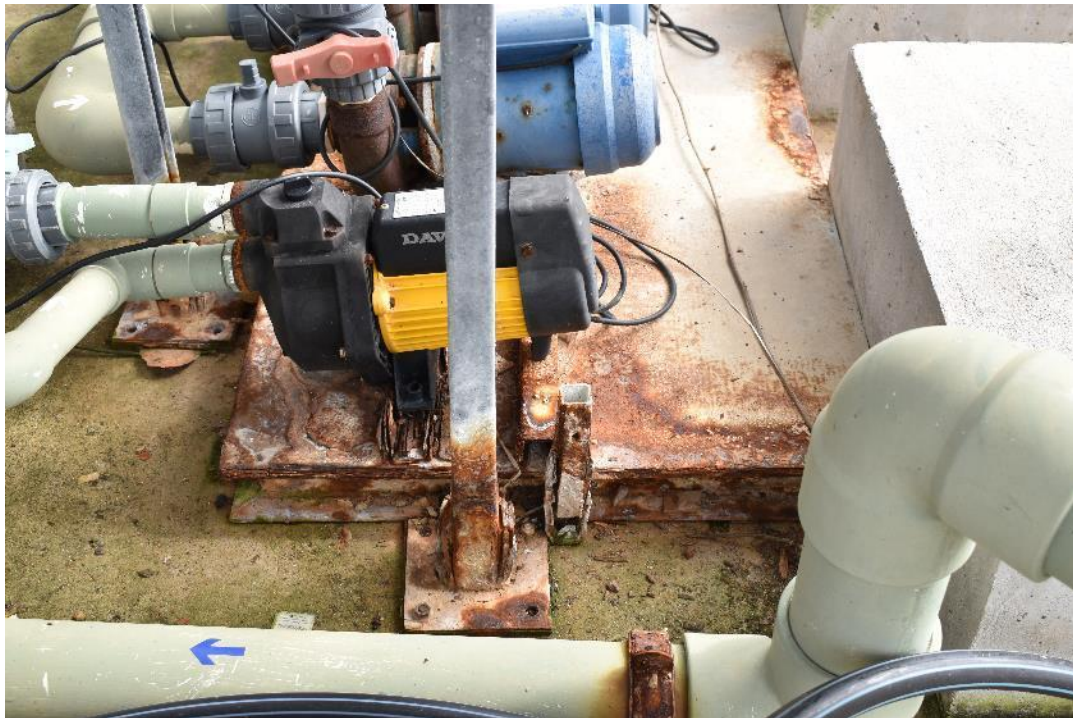
Figure 26 - Clarifier Sprinkler Pump
