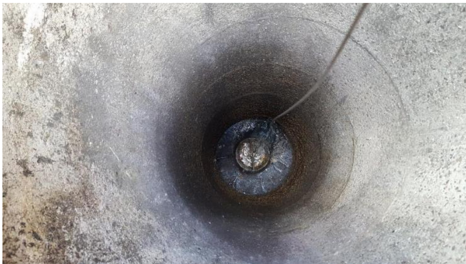
Figure 11 - SPS 1 Screening Manhole (Corrosion near invert)
