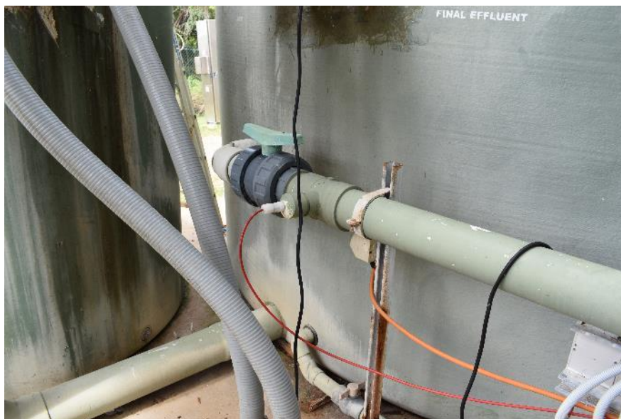
Figure 31- Sodium Hypochlorite dosing point
