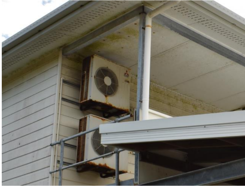
Figure 4 – Corroded Air-conditioning units & algal growth on roof
