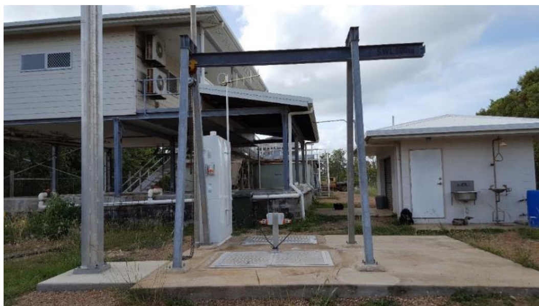
Figure 12 - Sewage Pump Station 1
