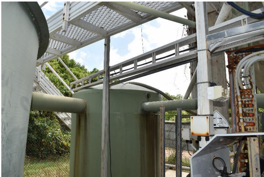
Figure 22 – Clarifier Lift Tank
