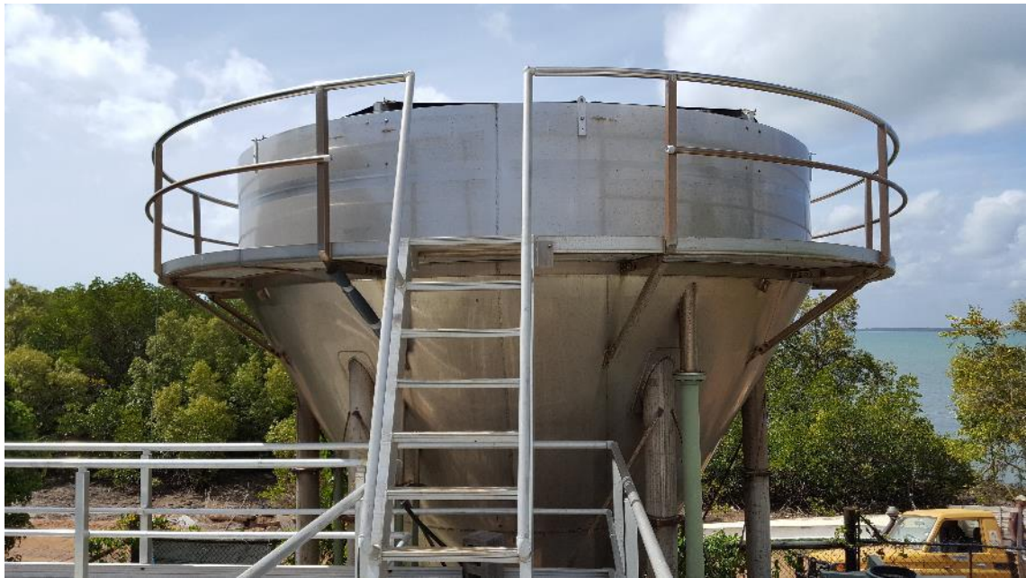
Figure 33 – Clarifier (missing handrailing)
