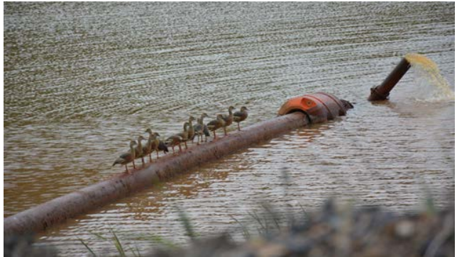
Photo 2.4 RD7 lime-dosing recirculation line
