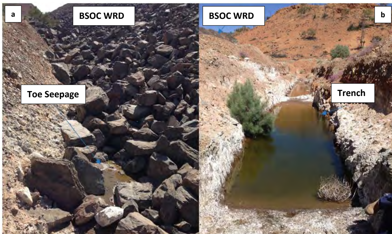
Figure 5-4: BSOC WRD South Seepage. a) Facing north, toe seepage behind the trench, b) Collection of seepage within the trench (facing south) (August, 2015)
