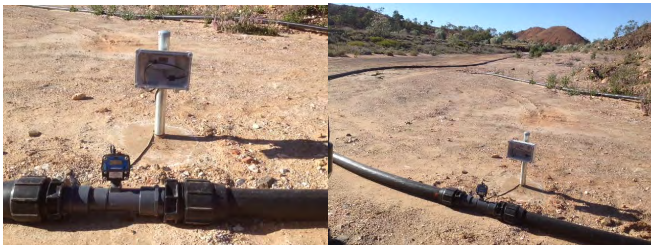
Figure 5-29: BSOC WRD South Seepage transfer pump flow monitoring equipment (June, 2016)
