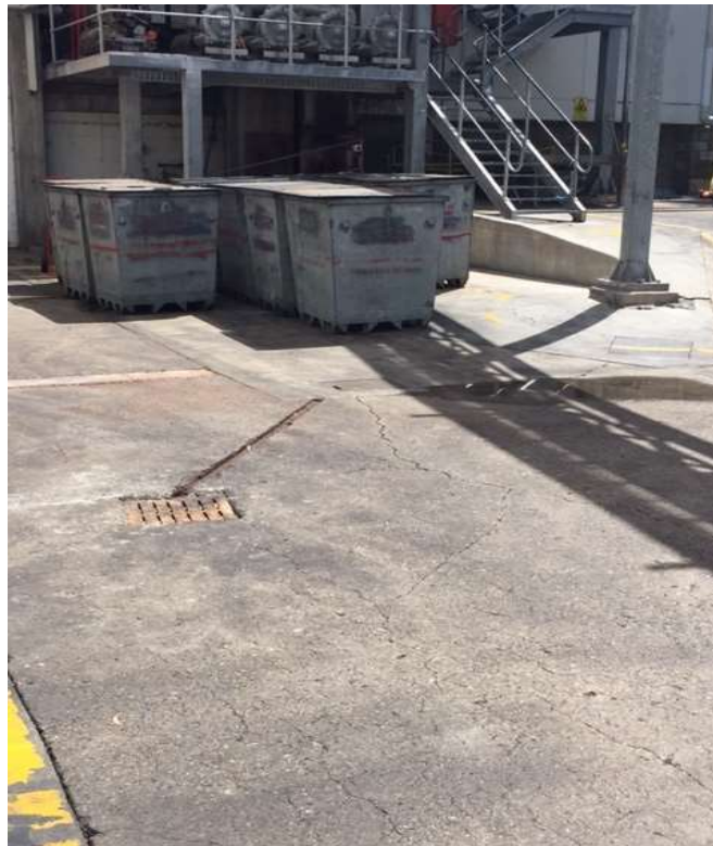
Figure 12 – Drains 6 (left), 5 (middle), 4 (right) and raw material bin causing potential contamination.
