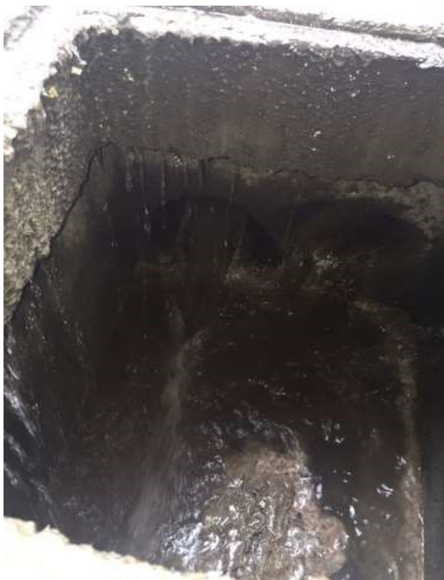
Figure 5 – Significant volume of stormwater entering stormwater drainage system during rain event. Believed to be from roof stormwater which is to be identified later in the report
