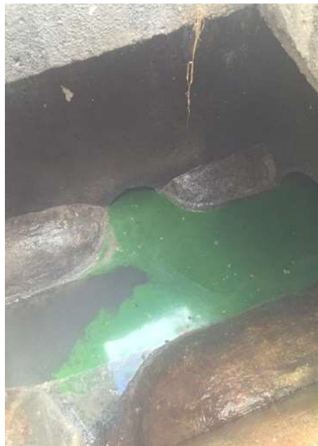
Figure 11 – Tracing Dye entering Drain 2 from Drain 4, 5 and 6.
