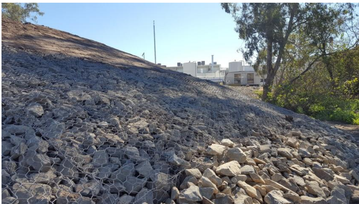
Figure 6: Installed scour protection on the eastern contaminated pond to maintain wall integrity during significant rainfall events.
