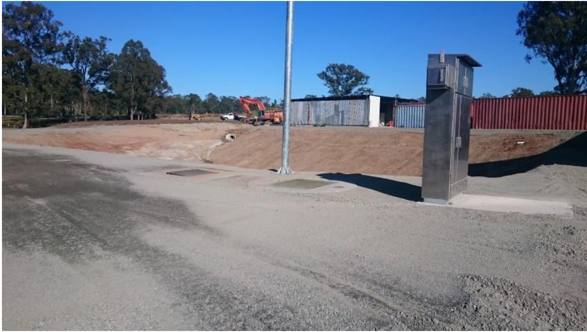
Figure 4: Installed control panel at the Eastern Stormwater Pond.
