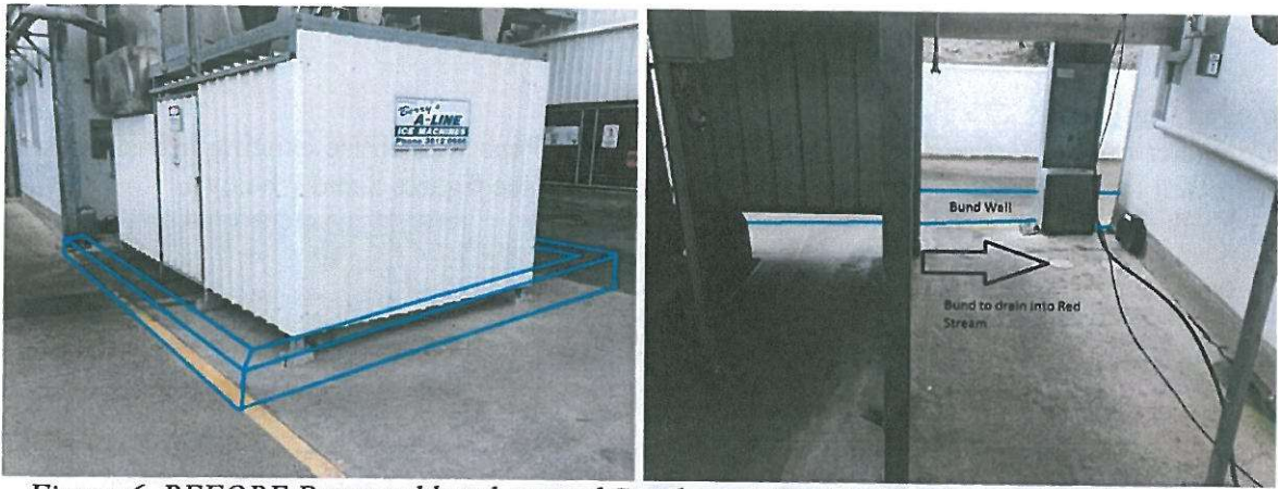
Figure 6. BEFORE Proposed bund around Steriliser Water Tank featured in TEP M6 Report.
