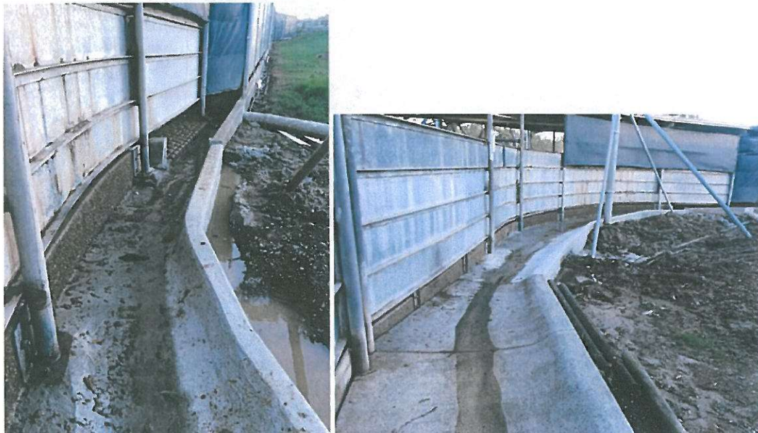
Figure 9 AFTER. Completion of the bunding on the eastern side of the cattle yard.
