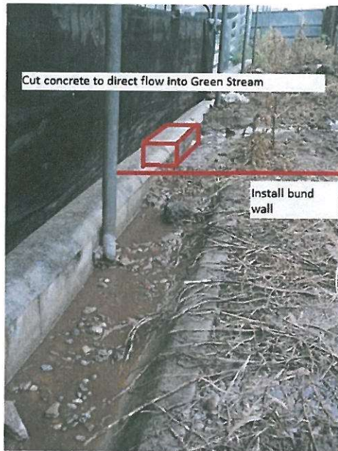
Figure 10. BEFORE Installation of concrete drain to divert all flow to the green stream.
