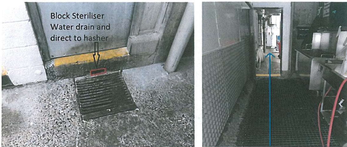
Figure 12. BEFORE Proposed Paunch Room Entry Steriliser Water Drain as featured in Figure 10 of M6 Report and Entry Steriliser Water Drain Diversion Path back to Hasher Room
