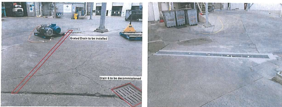
BEFORE and AFTER Installation of grated drain in hard stand area to capture potentially
