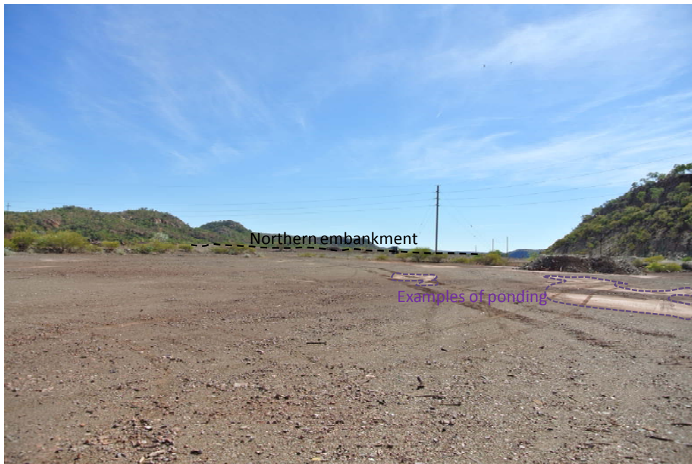
Figure 2.3 Old tailings storage facility examples of ponding
