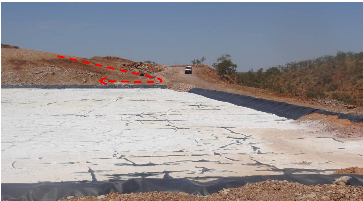
Earthworks to ensure contaminated water drains to pit and not Magazine Creek.
