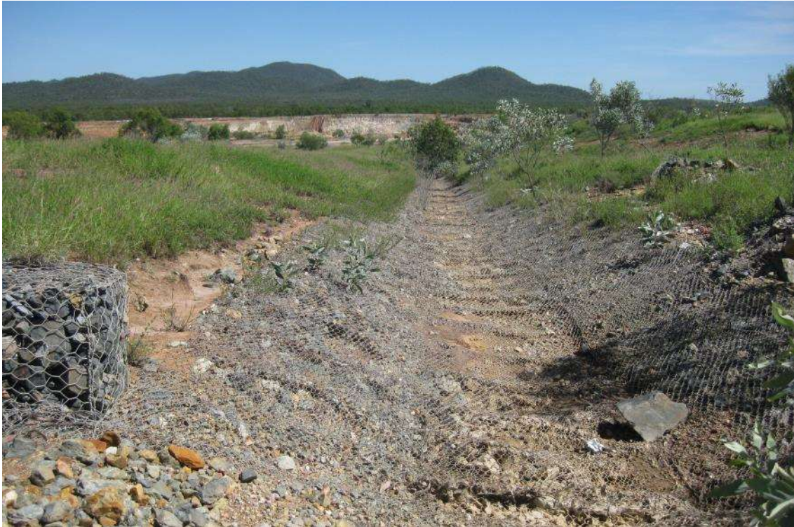
Main drain, east of pit. Rock filled gabion mattresses
