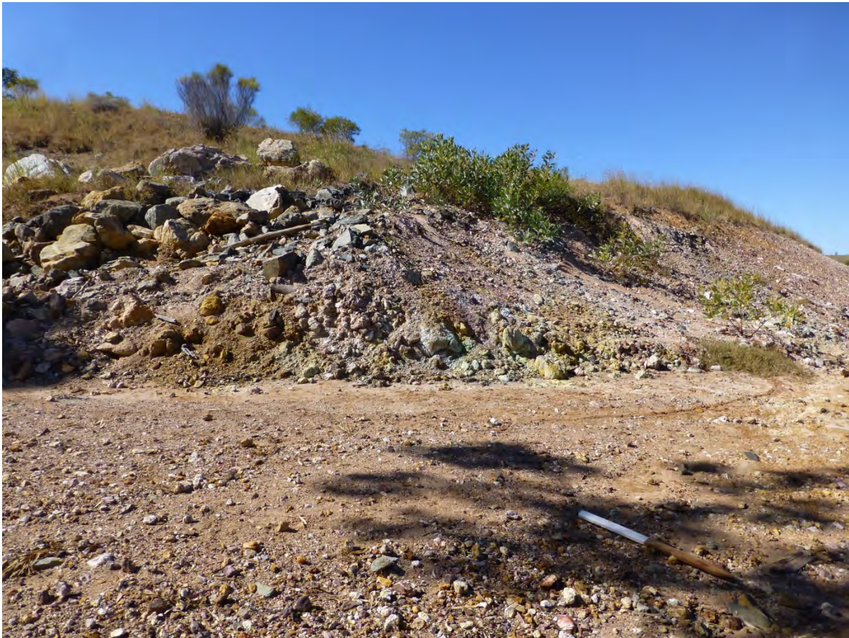
Figure 3 Potential Highway Waste Rock Dump Seepage
