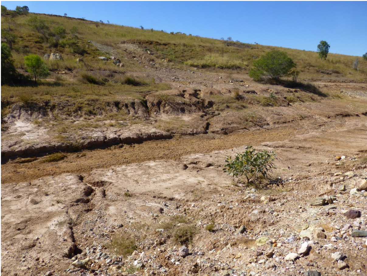
Figure 4 Eroded Structure with Exposed Sulphides
