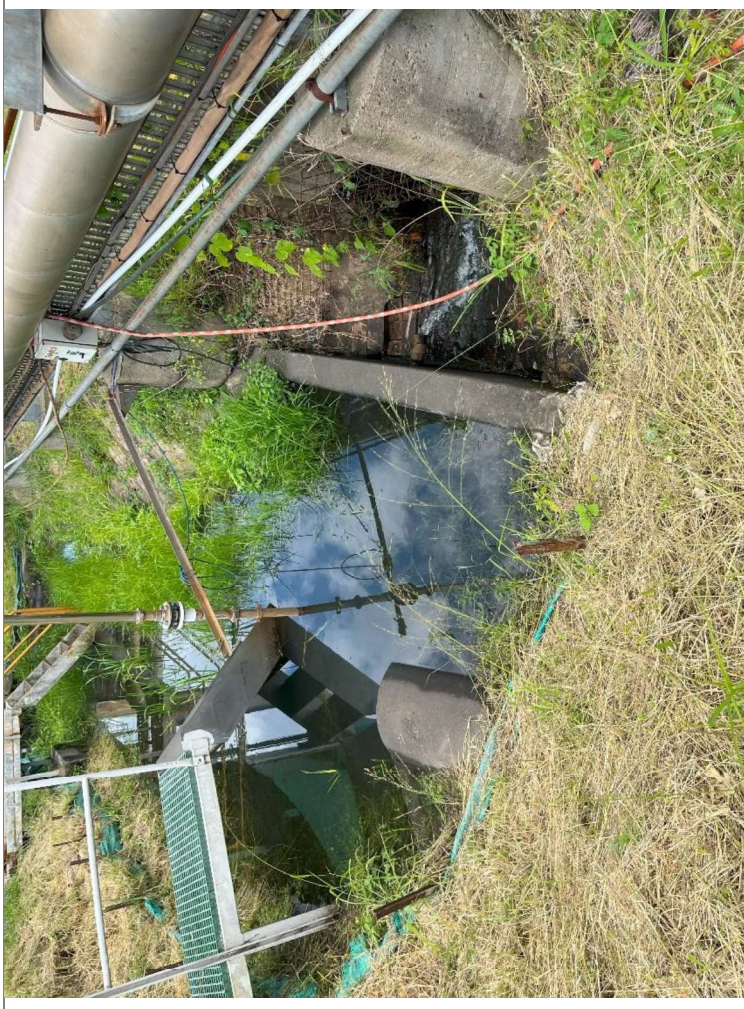
Photo 10: Stormwater first flush (2nd) manual valve open, pump running, and no water quality testing performed at time of site inspection. Image captured by the departmental officers, 3 January 2025.
