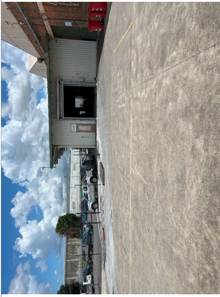
Photo 4: Bulk Chemical Storage building with carpark to left of image. Surface flow of acid evident across the concrete to the stormwater drains. Image captured by the departmental officers, 3 January 2025.
