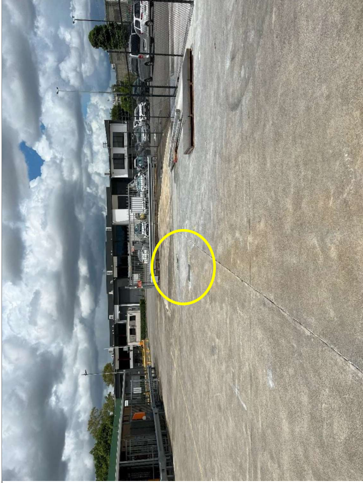
Photo 5: View to the west-southwest, the Bulk Chemical Storage building to right of image. Two stormwater surface drains present (circled). Acid etching from the event visible to the right of the image. Image captured by the departmental officers, 3 January 2025.
