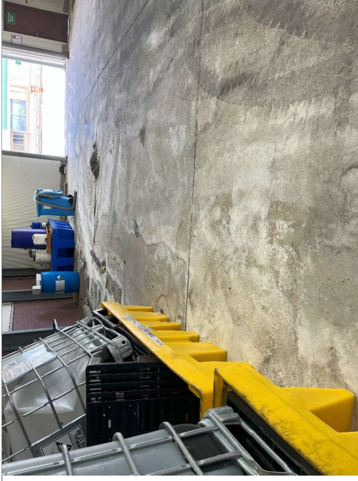
Photo 3: Bulk Chemical Storage building. Location of incident, absence of secondary bunding to prevent flow of chemicals. The floor is generally flat and grades towards the doorway. Image captured by the departmental officers, 3 January 2025.
