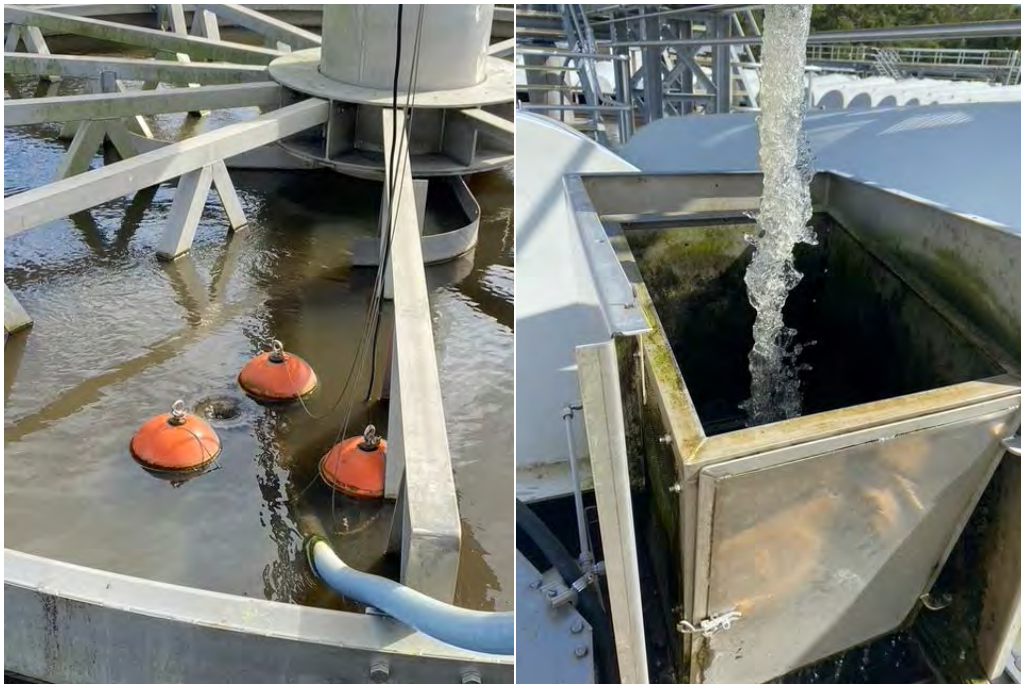
Figure 2: Clarifier Surface Skimming System (left photo shows surface skimming system and right photo shows 2mm screened collection container)
