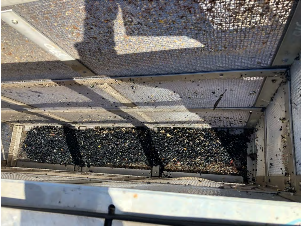
Figure 1 - Effluent Basket Screen with Captured MBBR Plastic Media Fragments (Aerial View)
