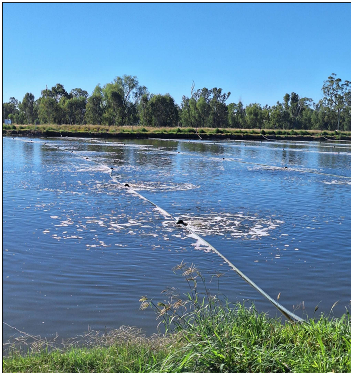
Figure 1: Photograph of desludged facultative lagoon and new aeration system installed and operating. Photo taken on the 24/06/2026.
