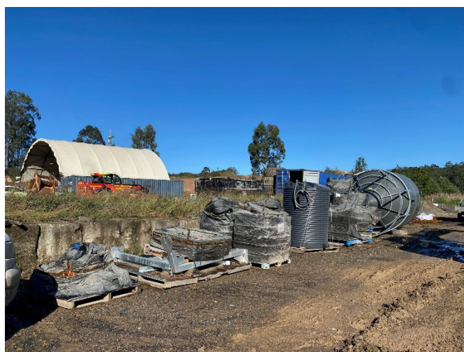
Figure 4 - Wheel wash and ancillary equipment as received on site
