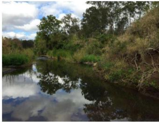
Figure 13: Typical eroded bank with only grass growing on it and no trees. This type of bank is highly prone to erosion in future flow events.
