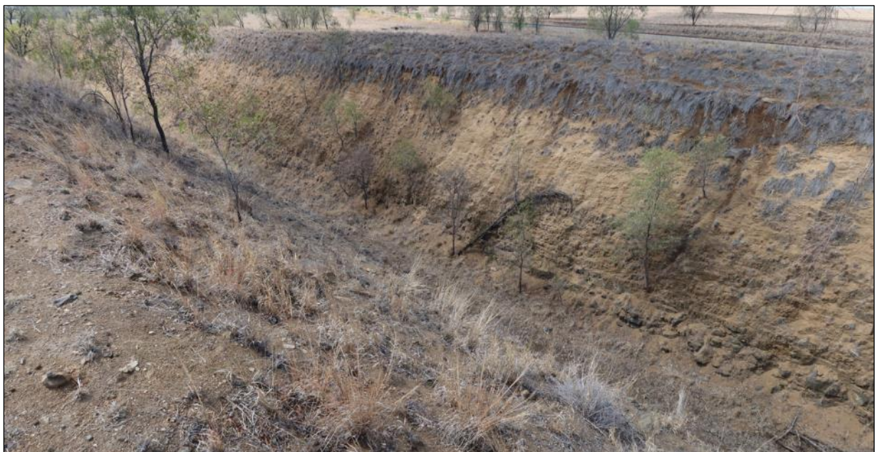
Figure 11-7 - Southeast (trapezoidal) channel cut in weathered basalt with nominal 2v:1h batters, local gullying, and opportunistic revegetation (view upstream towards north)
