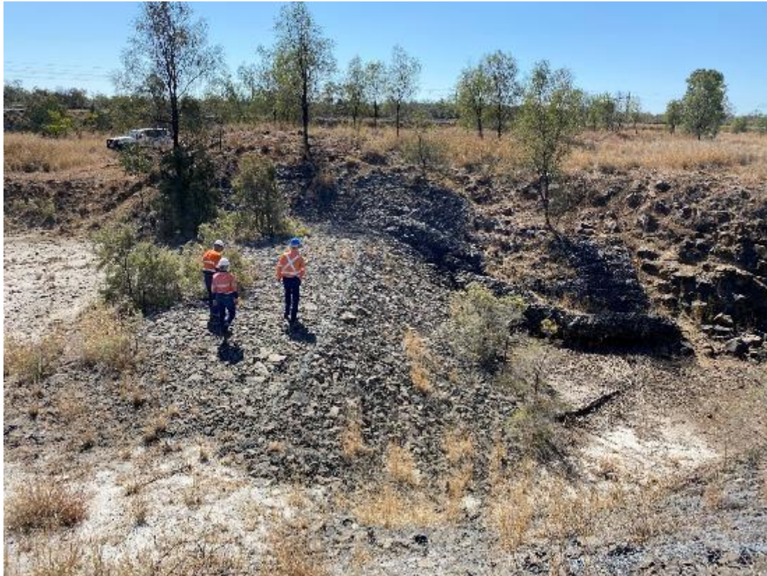
Figure 4-7 - Scour and instability at the diversion bywash
