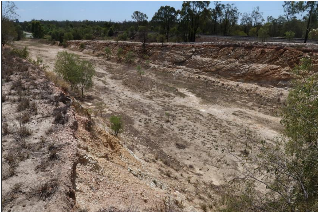
Figure 11-2 - West part of northwest channel cut viewed towards northwest showing erosion of batters in weathered Anakie Metamorphics and soil capping
