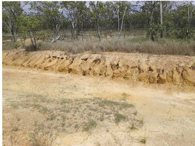
Plate 2: Erosion along TSF4 diversion drain banks, sediment deposition in drain invert
