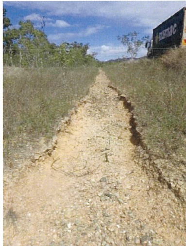
Plate 1: TSF4 diversion drain invert erosion with vegetated banks
