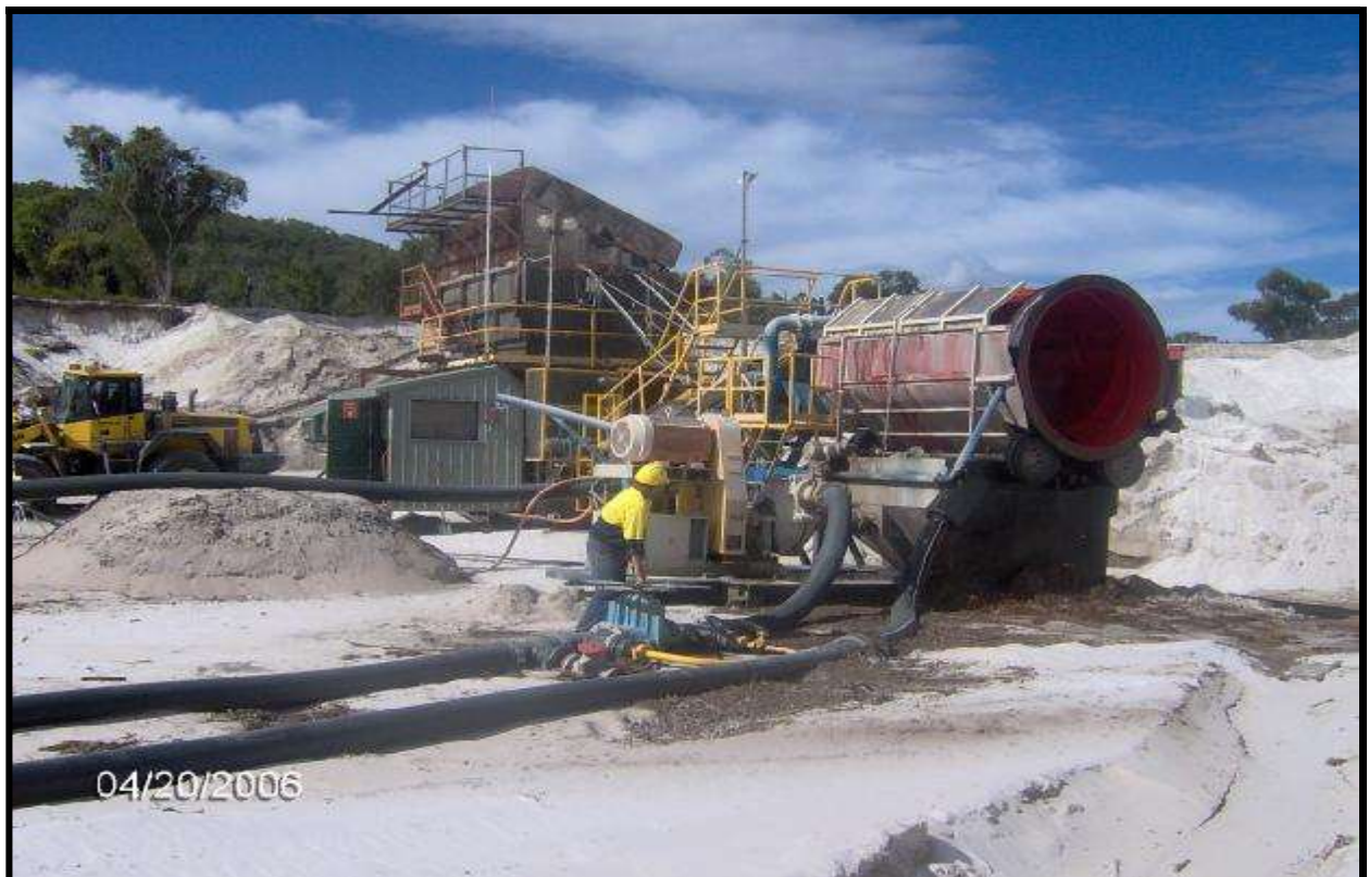
Photo 2. Primary Screening Plant
