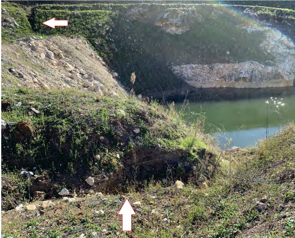
Figure 35. Two deep gullies cut in the haul-road and ramp at the west end of the East-West pit by water shedding off the ramp require remediation.
