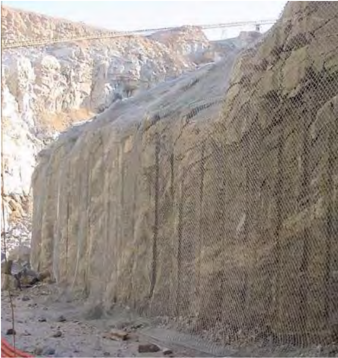
Figure 53. Example of a batter draped in high tensile strength rockfall mesh.
