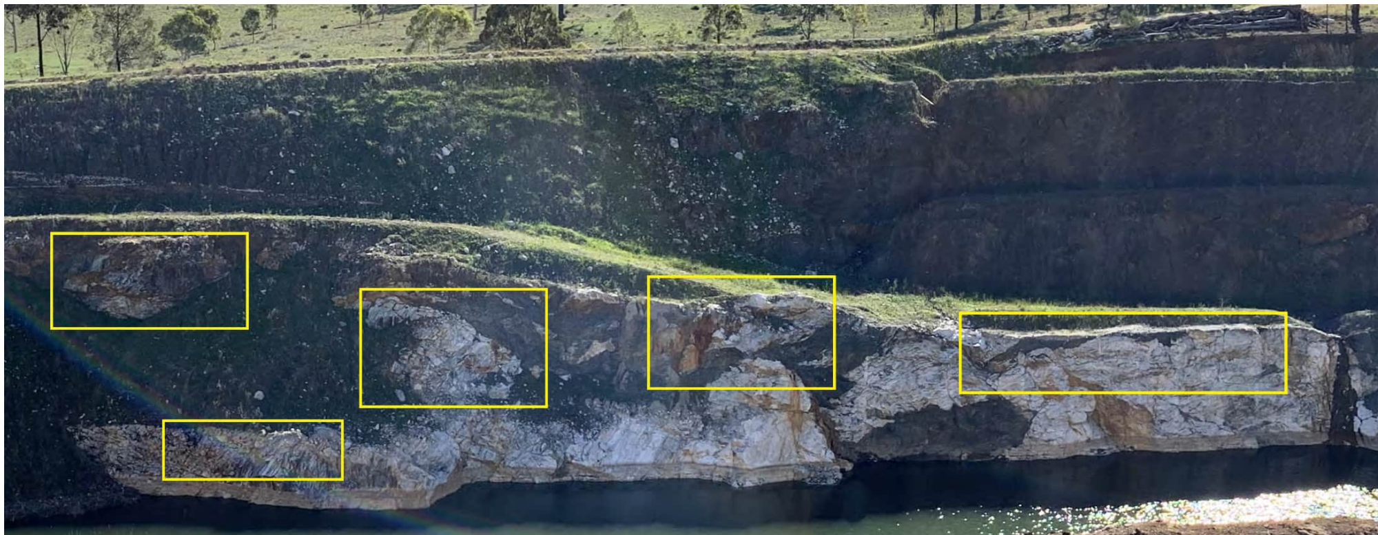
Figure 23. Loose and overhanging rocks (highlighted) on the batters of the north wall at the west end of the East-West pit.
