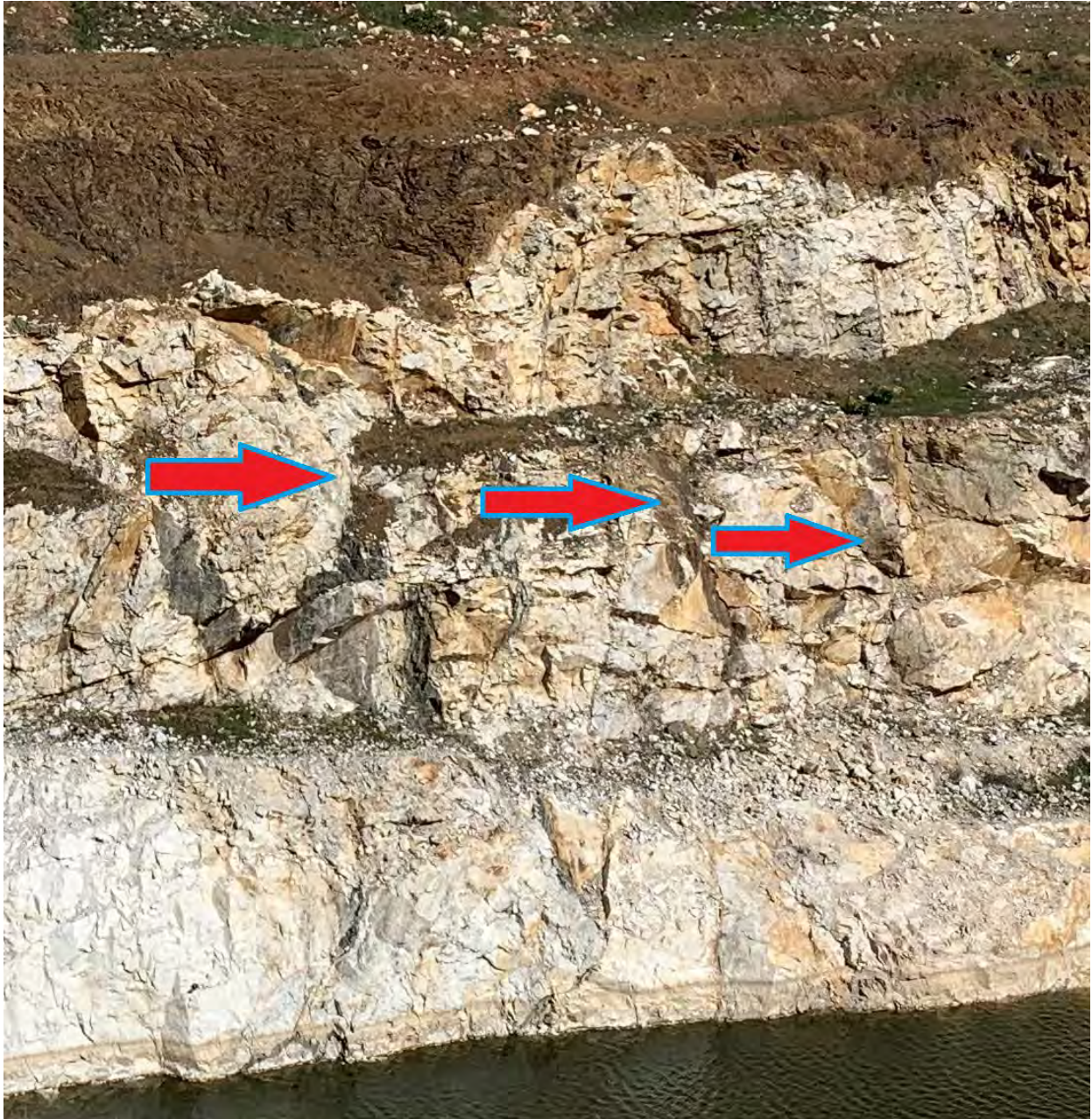
Figure 14. Examples on the south wall at the west end of the East-West pit of discontinuity spacings being significantly less than the mean values. The rock masses in these areas have accelerated weathering and localised instabilities that extend over multiple benches.
