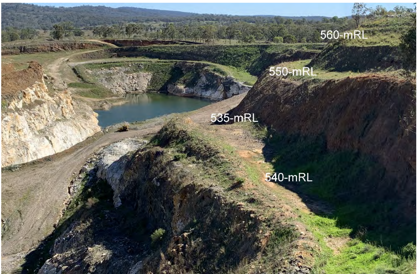
Figure 52. Water shedding off the 550-mRL berm is destabilising the 540-m to 550-mRL batter adjacent to the central ramp. Lined drains are required above and along the berm and down the batter.
