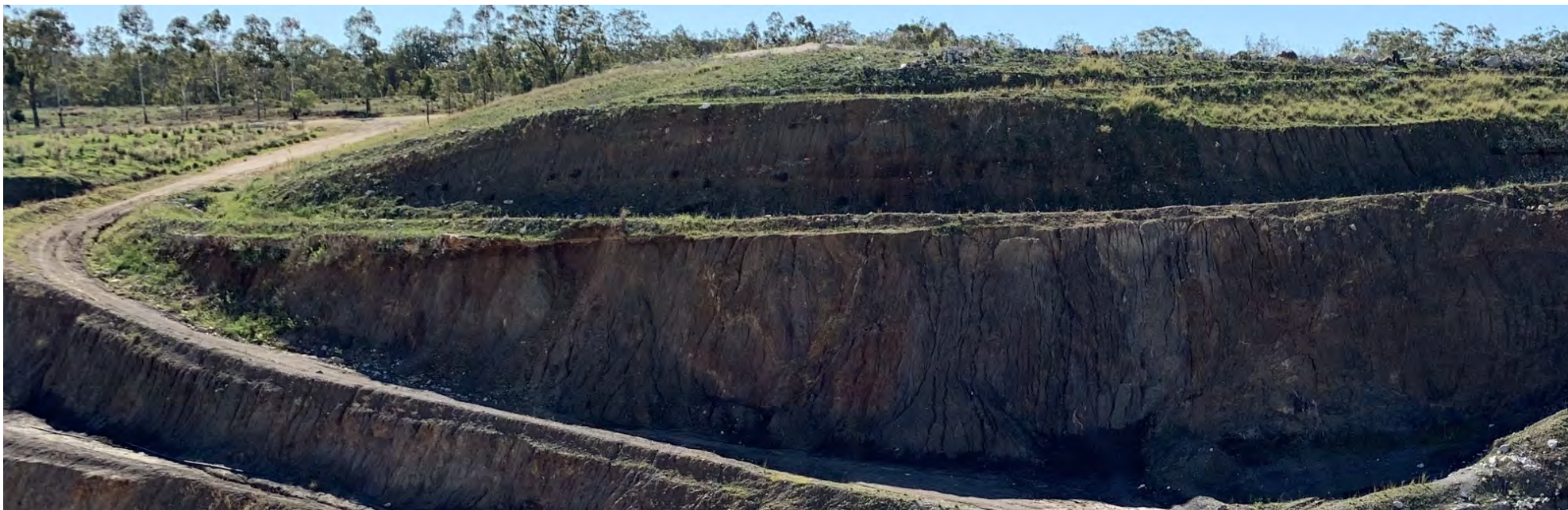
Figure 49. Batter adjacent to the central ramp in the East-West pit requires draped rockfall mesh and improved drainage on the ramp and 550-mRL berm above the ramp.
