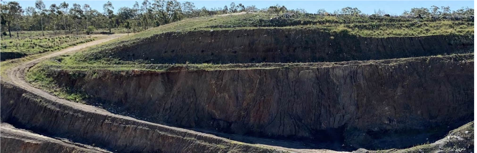
Figure 49. Batter adjacent to the central ramp in the East-West pit requires draped rockfall mesh and improved drainage on the ramp and 550-mRL berm above the ramp.
