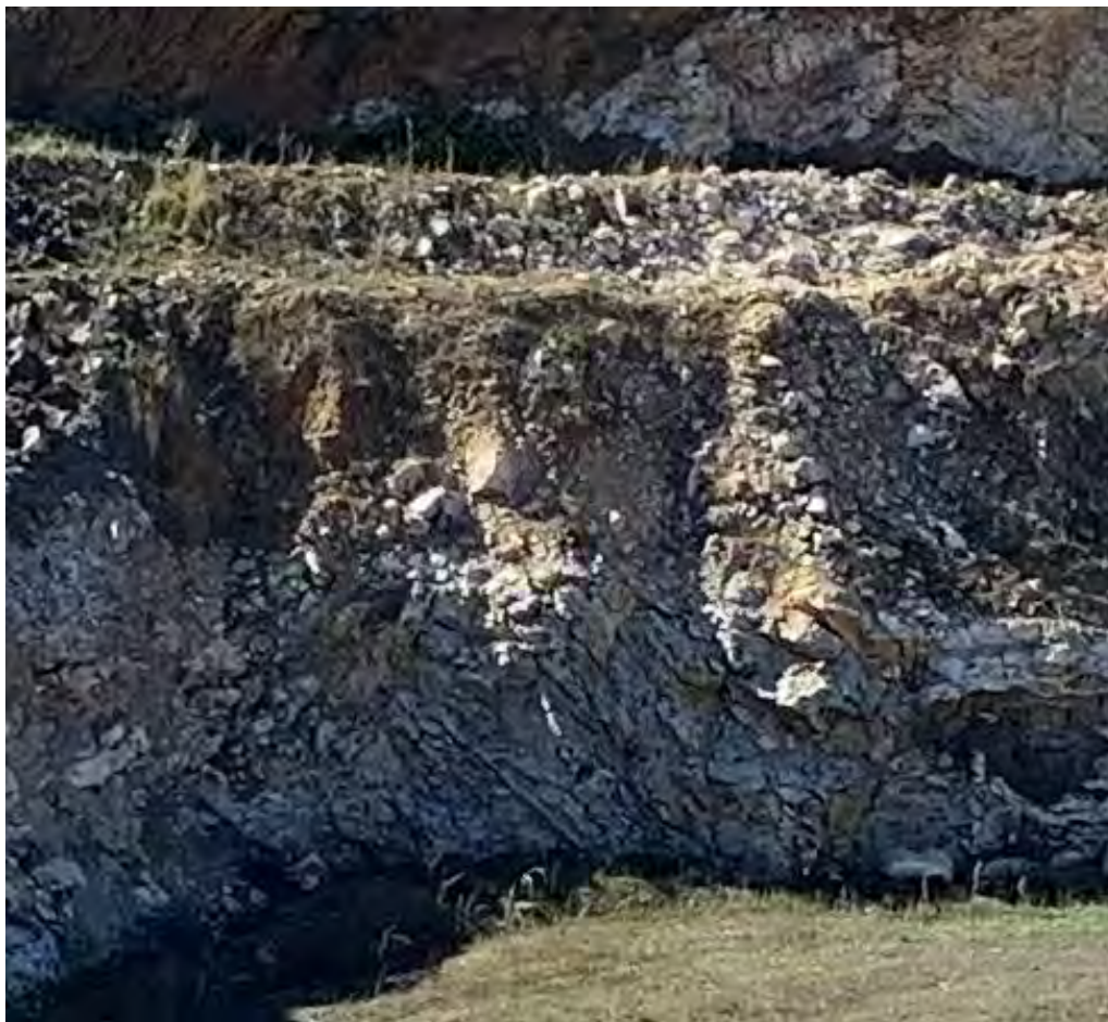
Figure 30. Sawtooth profile on the lower batter of the north wall of the east pit in the East-West pit due to multiple wedges sliding.
