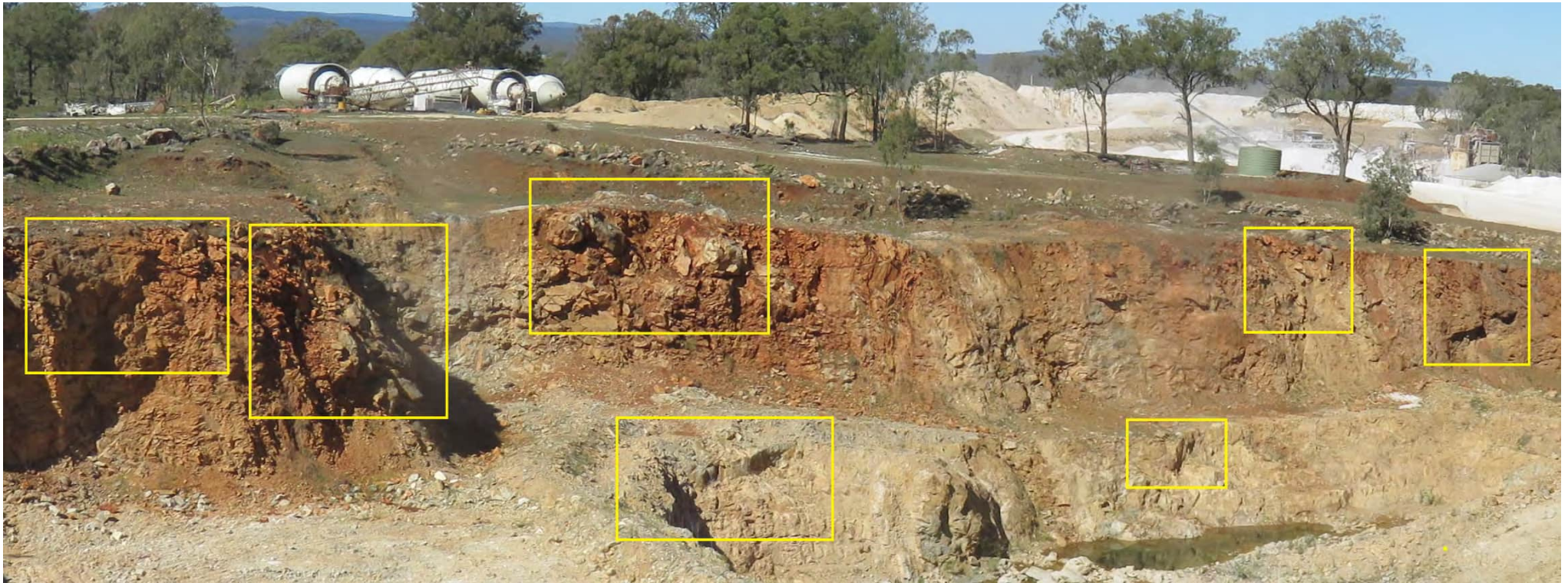
Figure 29. Loose rocks on the batters and overhanging rocks (highlighted) and loss of berm widths and scree on the berms on the east wall of the Aspal pit.
